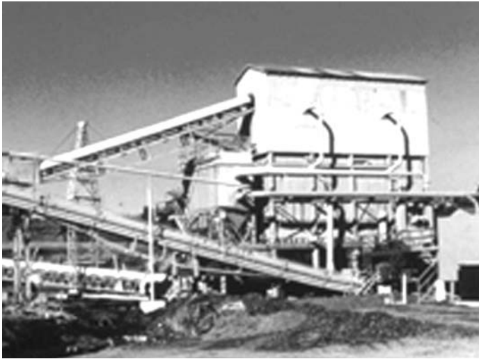
1.4 Equipment in sound-deadening, vacuum-equipped enclosure.
