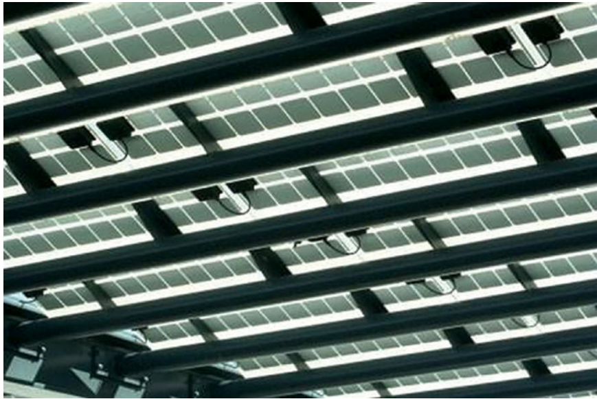
Figure 3.16 Ground, roof, and slate/tile mounted PV panels, Zurich Airport solar canopy (Photo by Steve Goodhew).
