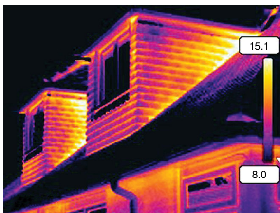
Figure 6.12 IR image of heat loss through dormer window structure (Photo by Steve Goodhew).
