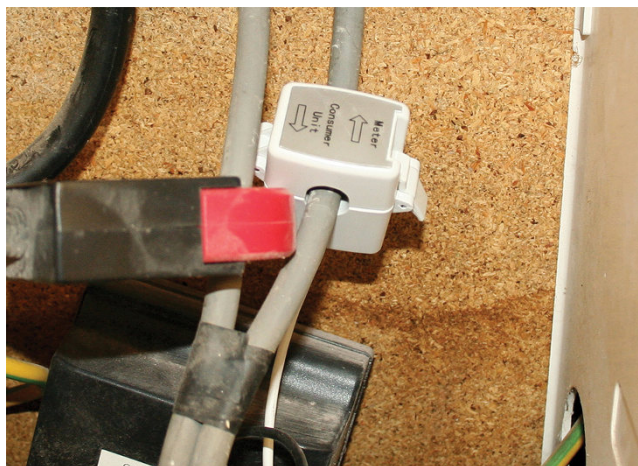
Figure 6.5 Clamps around electrical cables.
