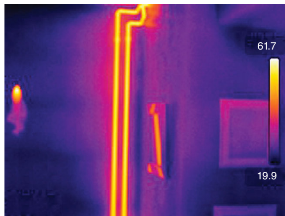
Figure 6.15 IR image of building services pipework (Photo by Steve Goodhew).
