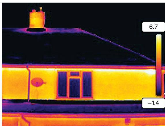
Figure 6.10 IR image of heat loss at roof ridge and chimney (Photo by Steve Goodhew).
