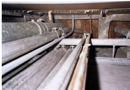
Electrical conduit risers, seen inside fire-resistance rated shaft, as seen entering bottom of a firestop. The firestop is made of firestop mortar on top, rockwool on the bottom. Raceways are used to protect cables from damage.
