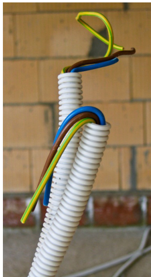
Colour-coded wires in a flexible plastic electrical conduit found commonly in modern European houses
