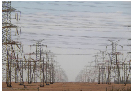
Transmission lines transmit power across the grid .
