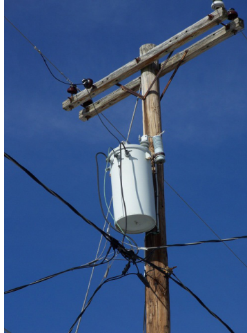
US single-phase residential power distribution transformer, showing the two insulated “Line” conductors and the bare “Neutral” conductor (derived from the earthed center-tap of the transformer). The distribution supporting centenaries are also shown.
