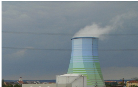
“Camouflaged” natural draft wet cooling tower
