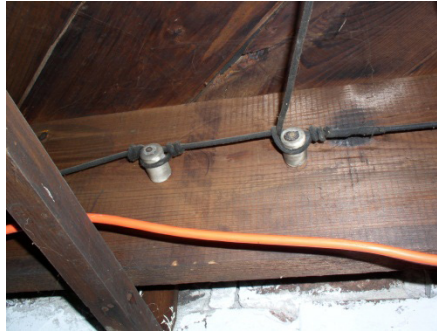
Knob-and-tube wiring (the orange cable is an unrelated extension cord)
