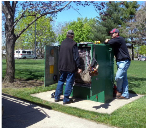
Engineers working on a cross-connect box, also known as a serving area interface.
