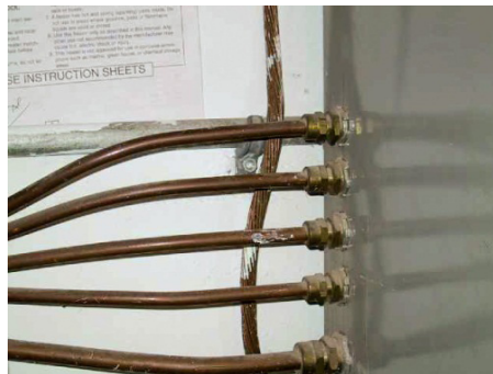
Mineral insulated cables at a panel board
