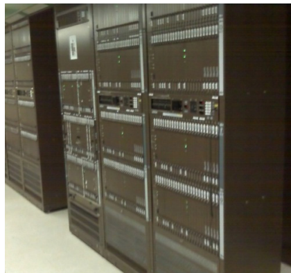
Typical Northern Telecom DMS100 Telephone Central Office Installation
