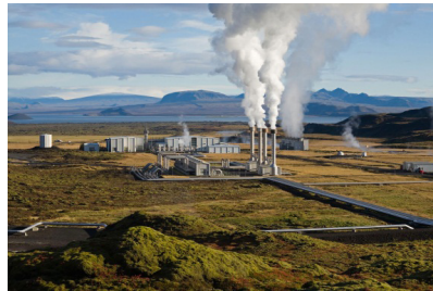
Nesjavellir Geothermal Power Station, Iceland.
