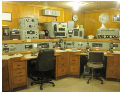
Radio Transmitter room
