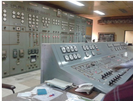
Control room of a power plant
