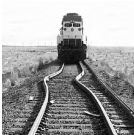
Figure 1.10 Rail thermal compression-induced track buckle. (Data from Kish, 1997.)
