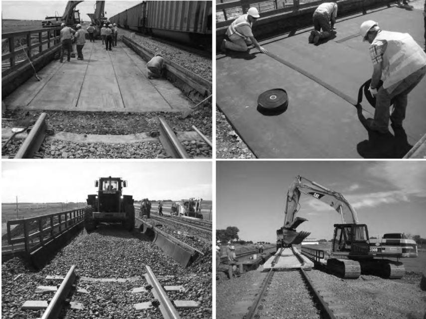
Figure 5.38 Installation of ballast mats in a heavy axle load and high-tonnage bridge in western United States.
