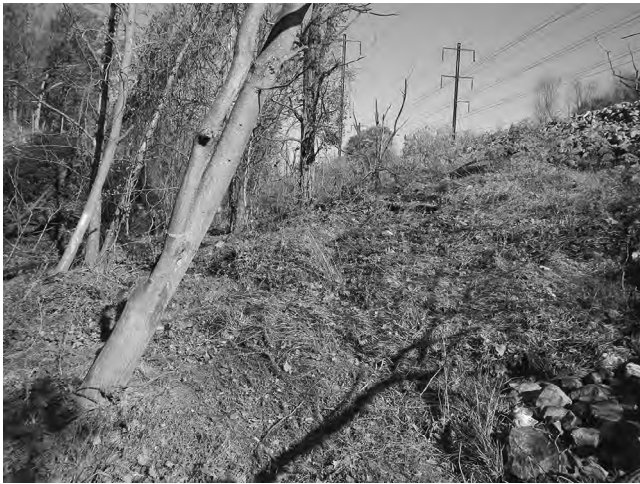
Figure 10.24 Backward tilting of trees and soil bulge at the toe of slope.
