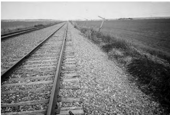
Figure 1.17 Embankment settlement problem.
