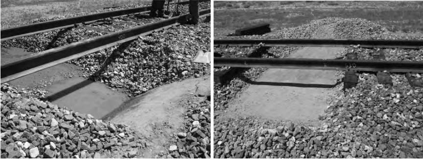
Figure 5.28 Left—Damaged asphalt and standing water. Right—Nearby undamaged asphalt.
