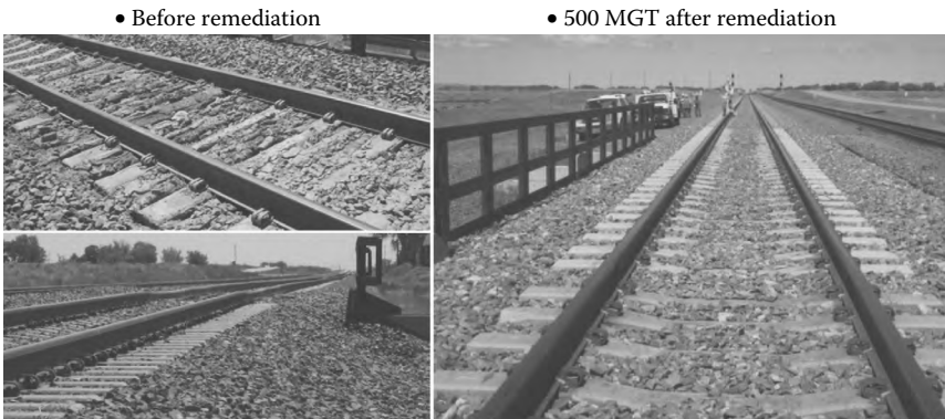
Figure 5.39 Improvement of track conditions from reducing track stiffness, increasing track damping, and track drainage accommodation.
