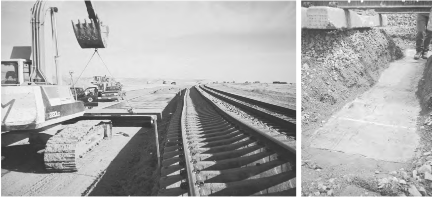
Figure 10.8 Geomembrane placement (left), and geomembrane after being in service for 200 MGT (right).
