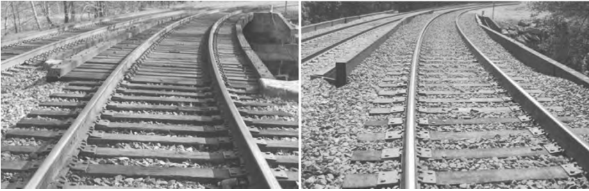
Figure 5.42 Change of open deck to ballast deck to achieve consistent track strength and restraint.
