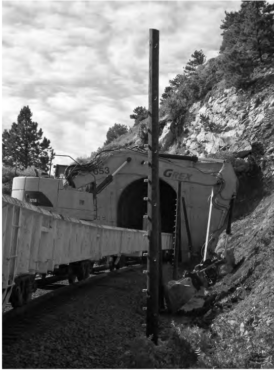
Figure 6.51 A “slot train” excavating a ditch. (Courtesy of Georgetown Rail Equipment, Georgetown, Texas.)
