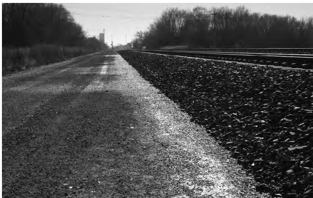
Figure 6.35 Poor internal drainage due to the long drainage path of a subballast that extends through the right-of-way road.
