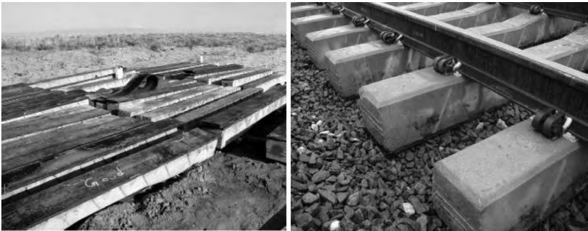
Figure 5.33 Concrete ties fitted with rubber pads on the bottom.
