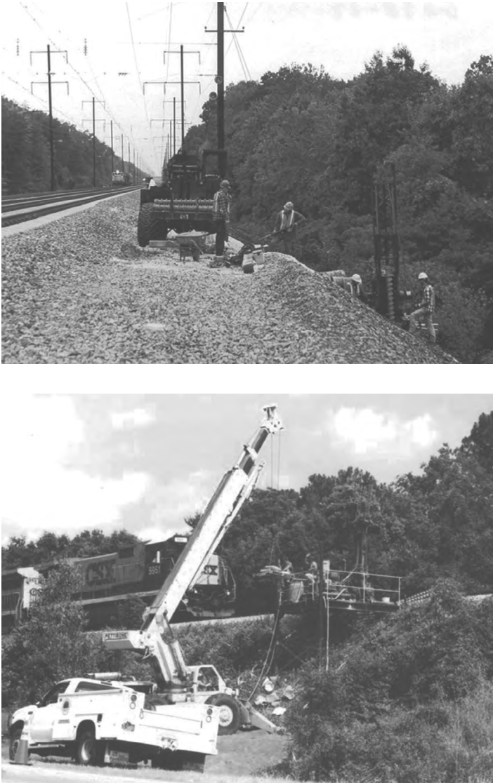
Figure 7.15 Drilling at crest and at midslope of a railway embankment (top). Drilling on a railway embankment using specialized drilling platform and crane (bottom). (Data from Hyslip, J. et al., Railway embankment assessment and case studies. Proceedings of International Heavy Haul Association Specialty Conference , Calgary, Canada, 2011.)
