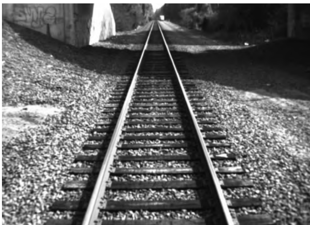
Figure 10.19 Example of poor external track drainage.
