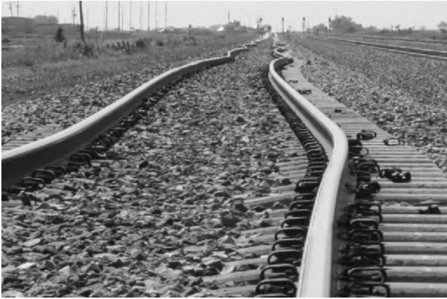
Figure 8.71 Example of continuous track buckling over extended track length.
