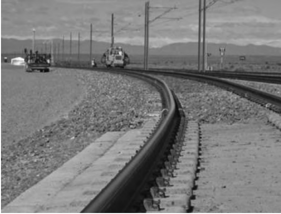
Figure 1.30 Ballasted track to slab track transition with alignment error.
