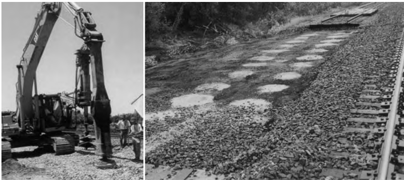
Figure 5.44 Use of stone columns to strengthen weak subgrade in the bridge approach.
