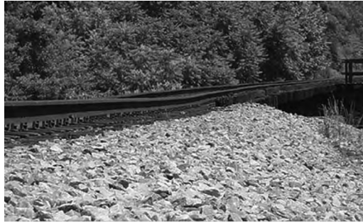
Figure 1.28 Track geometry deviation from transition settlement.
