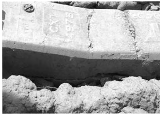
Figure 1.21 Concrete tie showing horizontal split on side and vertical cracks.
