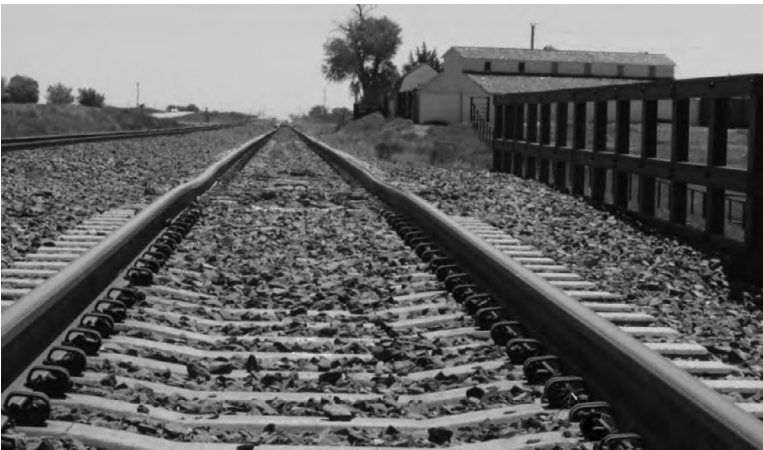
Figure 3.23 Dip at bridge transition.
