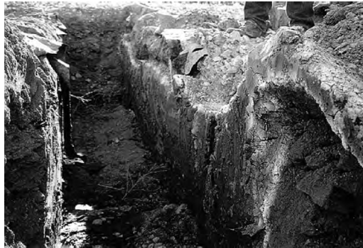
Figure 1.16 Progressive subgrade deformation.
