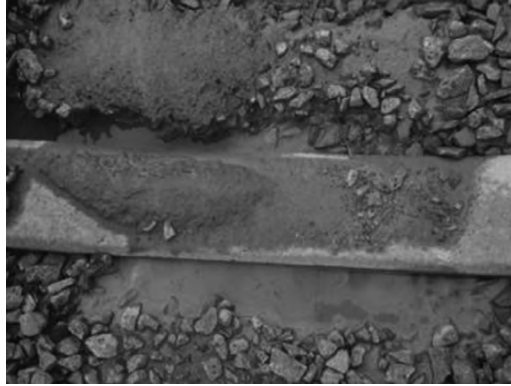
Figure 1.20 Concrete tie with fouled ballast that often results in a tie cavity.
