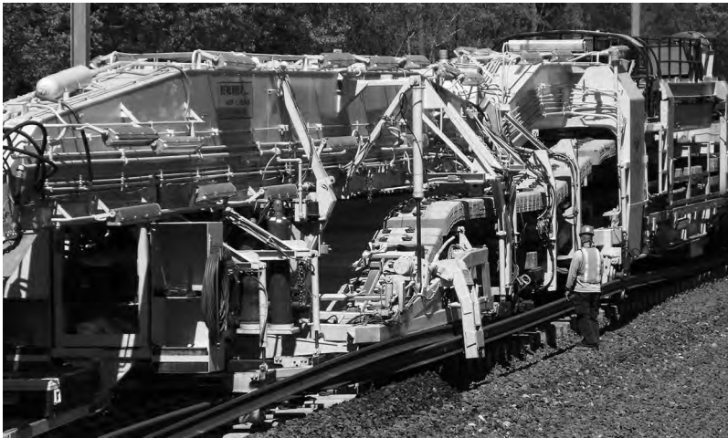
Figure 9.3 Close-up view of TLM placing new concrete ties and new rail. (Courtesy of Amtrak, Philadelphia, Pennsylvania.)
