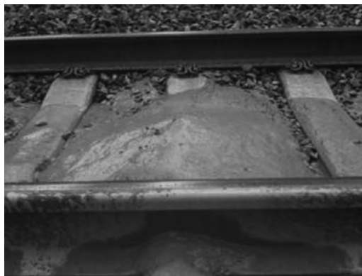
Figure 1.19 Ballast mud boil.
