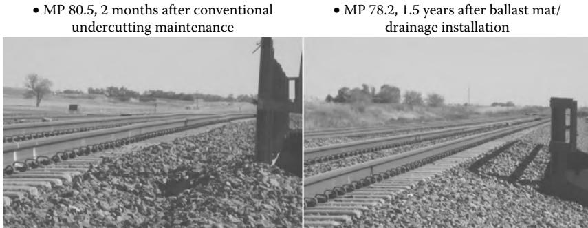
Figure 5.40 Comparison of track geometry condition for two nearby bridges with different maintenance practices.
