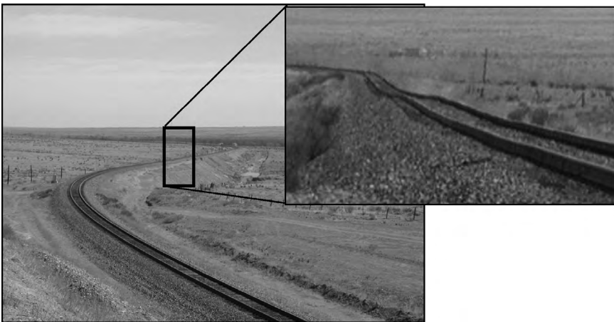
Figure 3.19 Track settlement zone due to weak subgrade.
