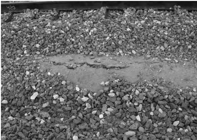
Figure 5.27 Early indication of asphalt failure.
