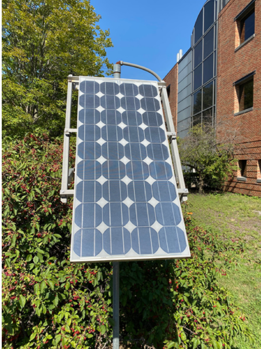
Figure 8.7 A solar panel.
