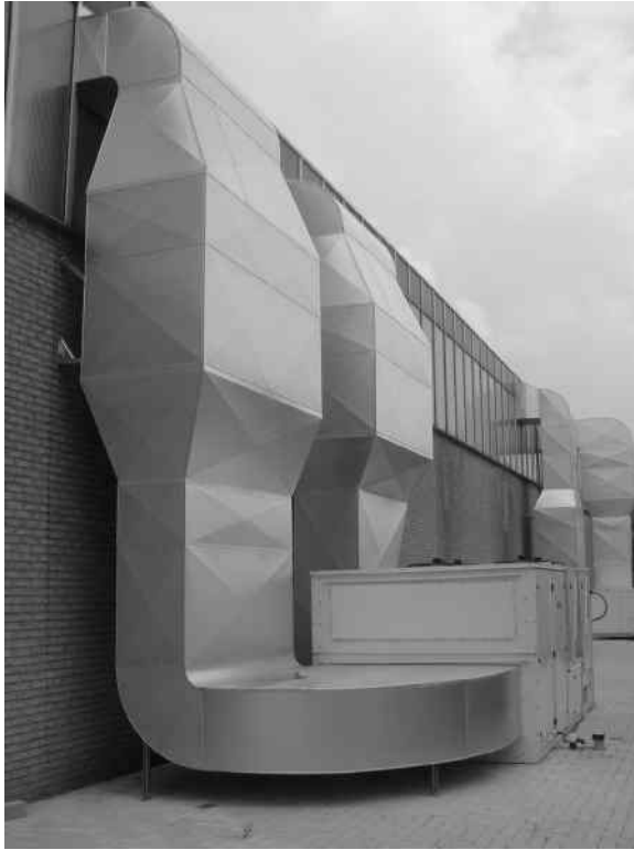
Figure 24.4 Air handling units providing air conditioning for production plant, total installed capacity 145 kW (Johnson Controls).
