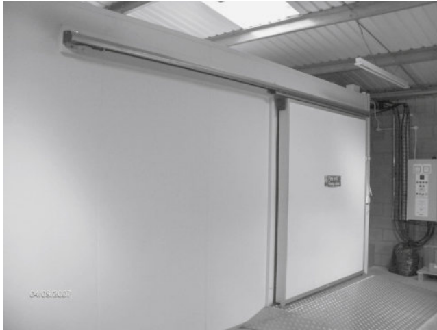
Figure 15.5 Sectional cold room (Michael Boast).
