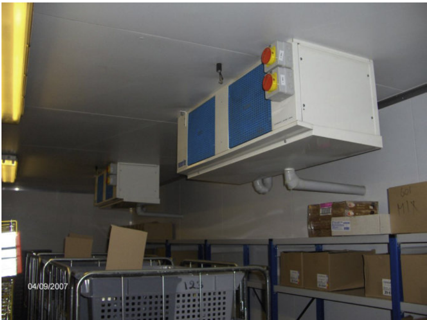
Figure 15.7 Ceiling-mounted coolers (Michael Boast)
