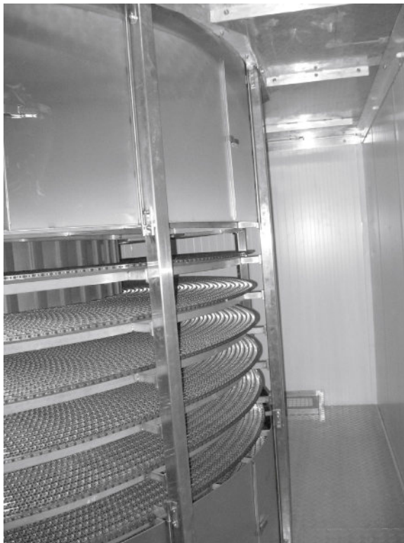
Figure 14.2 View of spiral freezer (Star Refrigeration).
