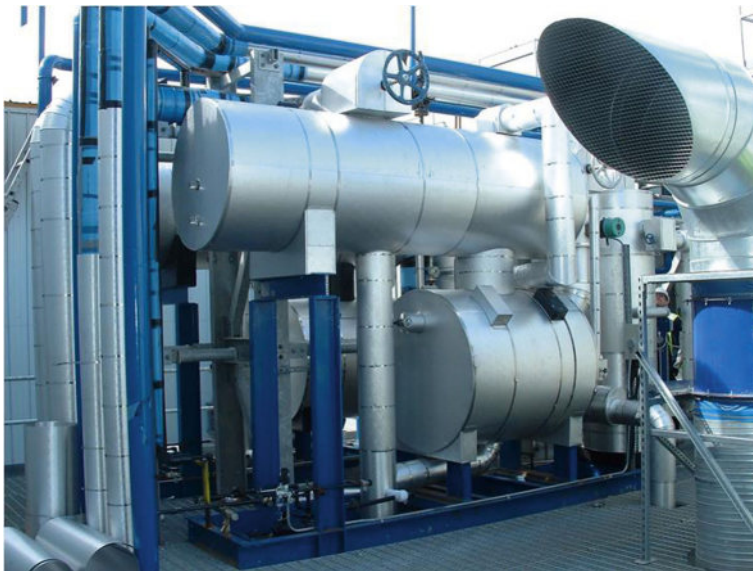
Figure 18.1 Condenser cascade (Star Refrigeration).
