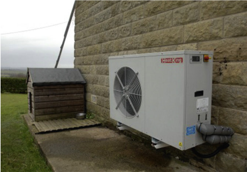
Figure 25.5 Wall mounted ASHP delivering 8 kW heating to a farmhouse (HeatKing).
