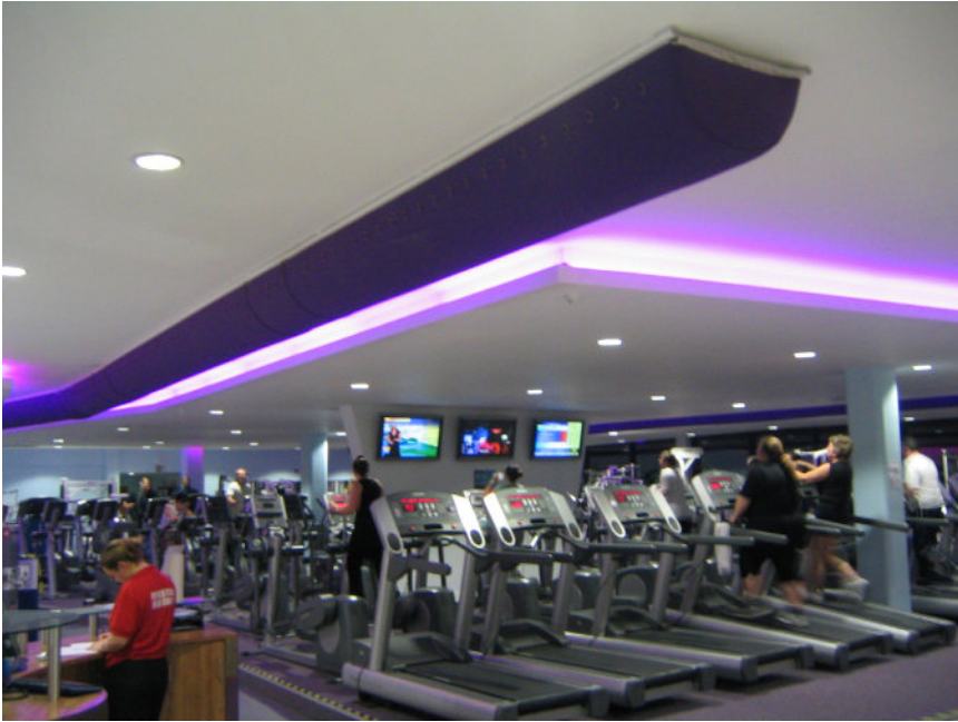
Figure 23.19 Textile ducting providing air distribution in a fitness centre (Business Edge).
