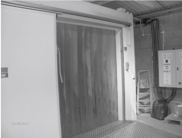
Figure 15.6 Cold room loading door open and strip curtain (Michael Boast).
