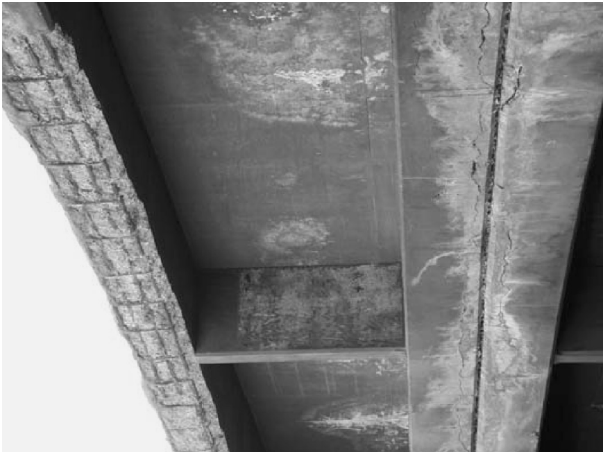
Figure 4.7 Example of steel corrosion.
