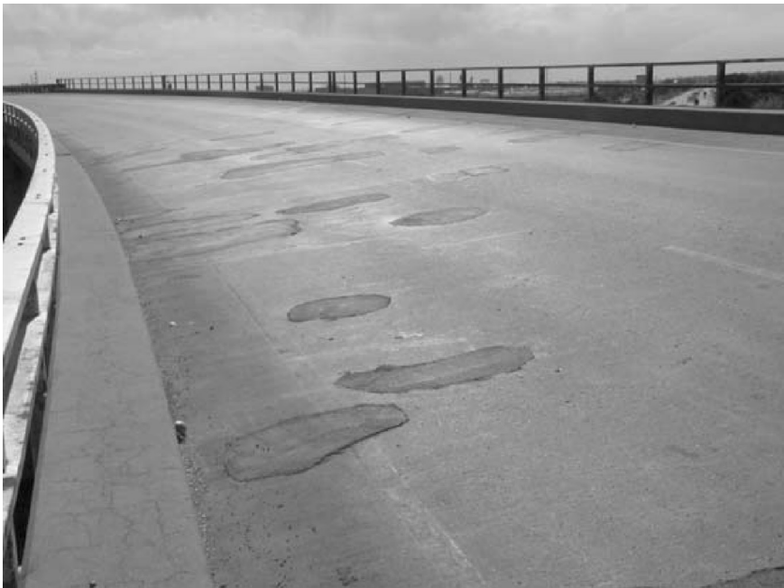
Figure 4.9 Many small patches applied on a bridge deck.
