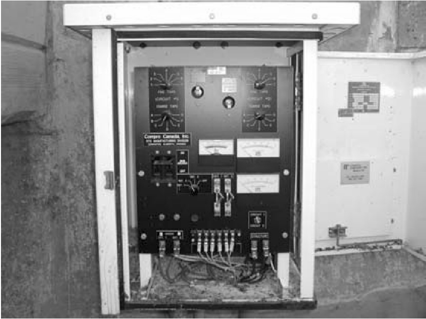
Figure 4.27 The control box for an impressed current cathodic protection system.
