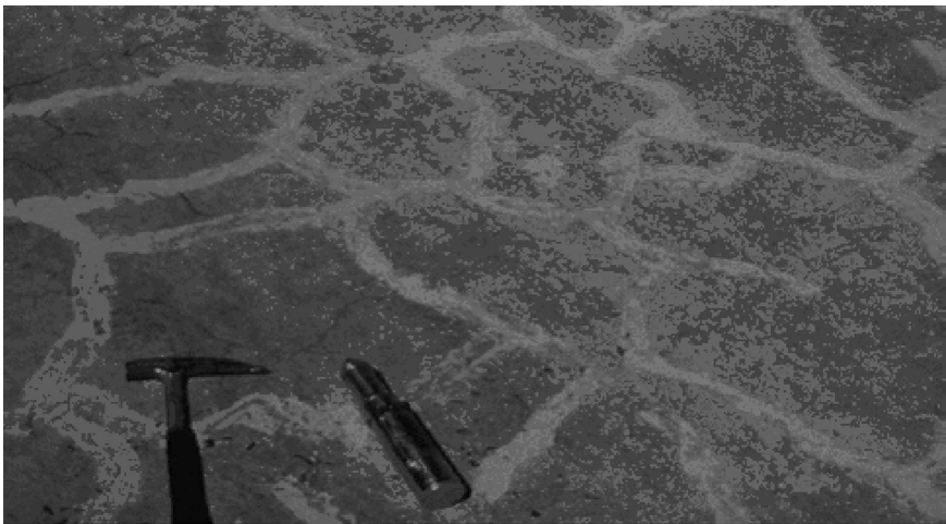
Figure 4.11 Appearance of a repaired concrete by improper crack repair techniques.
