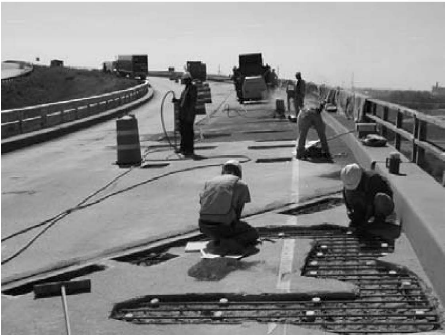
Figure 4.25 A sacrificial anode cathodic protection system, called Galvashield cathodic protection system was installed in SH 85 SB in Greeley, Colorado.
