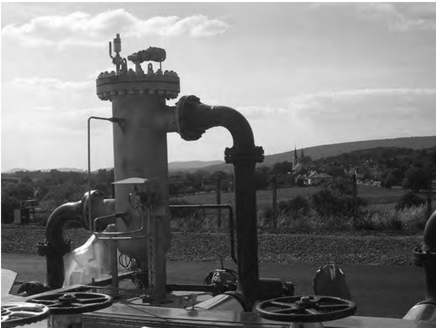
Figure 11.10 Soutz EGS power plant Source: EGEC (2008)
