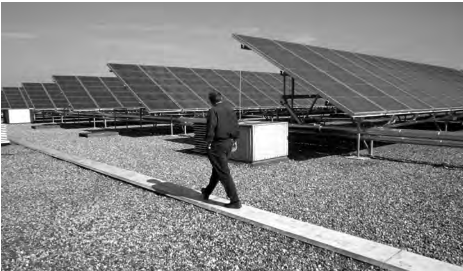
Figure 2.15 Collector field on the roof of a commercial building. Source: ZEN-International
