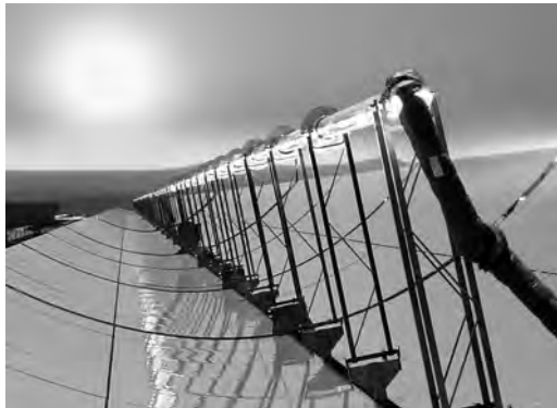
Figure 7.1 Parabolic trough plants
