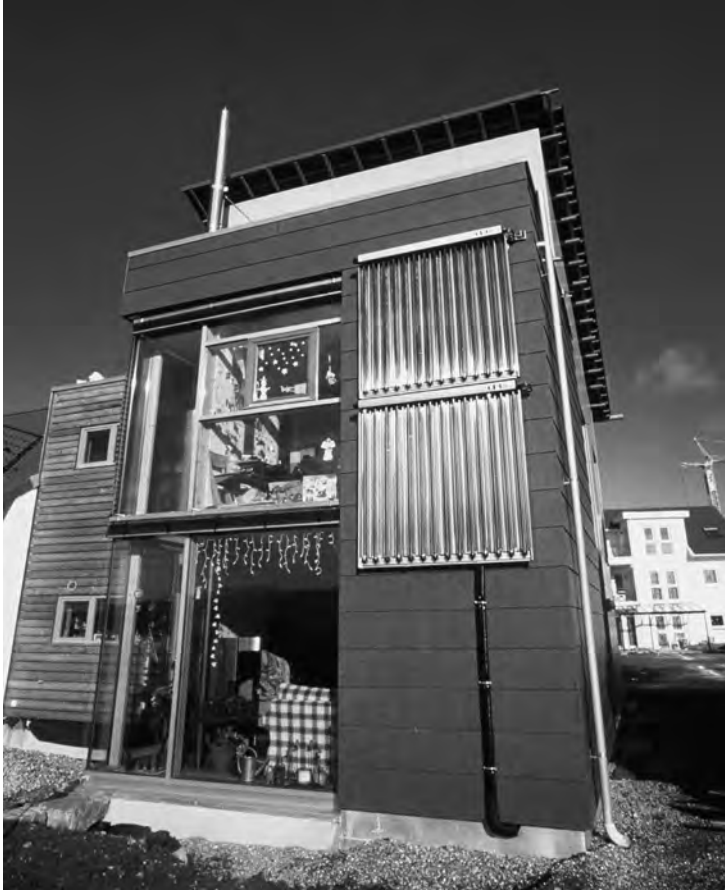
Figure 2.13 House with vacuum tube collectors installed on the facade Source: Ritter Solar
