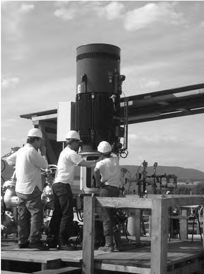
Figure 11.9 Soutz EGS power plant Source: EGEC (2008)
