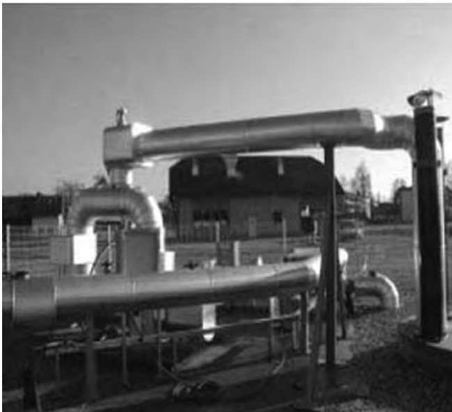
Figure 11.5 Altheim CHP: Well-head and pump station Source: EGEC (2008)
