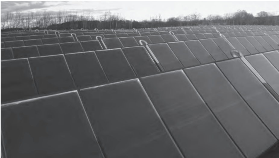
Figure 2.1 Solar heating and biomass plant, 5500 m 2 , Falkenberg, Sweden Source: ARCON Solvarme
