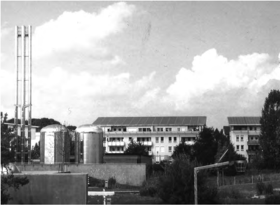
Figure 4.12 Solar collectors and buffer storage for small DH network with BTES
