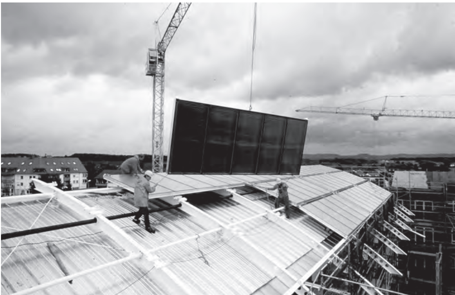
Figure 2.9 Large (custom-built) flat-plate collector being lifted/installed on roof in Germany Source: ARCON Solvarme
