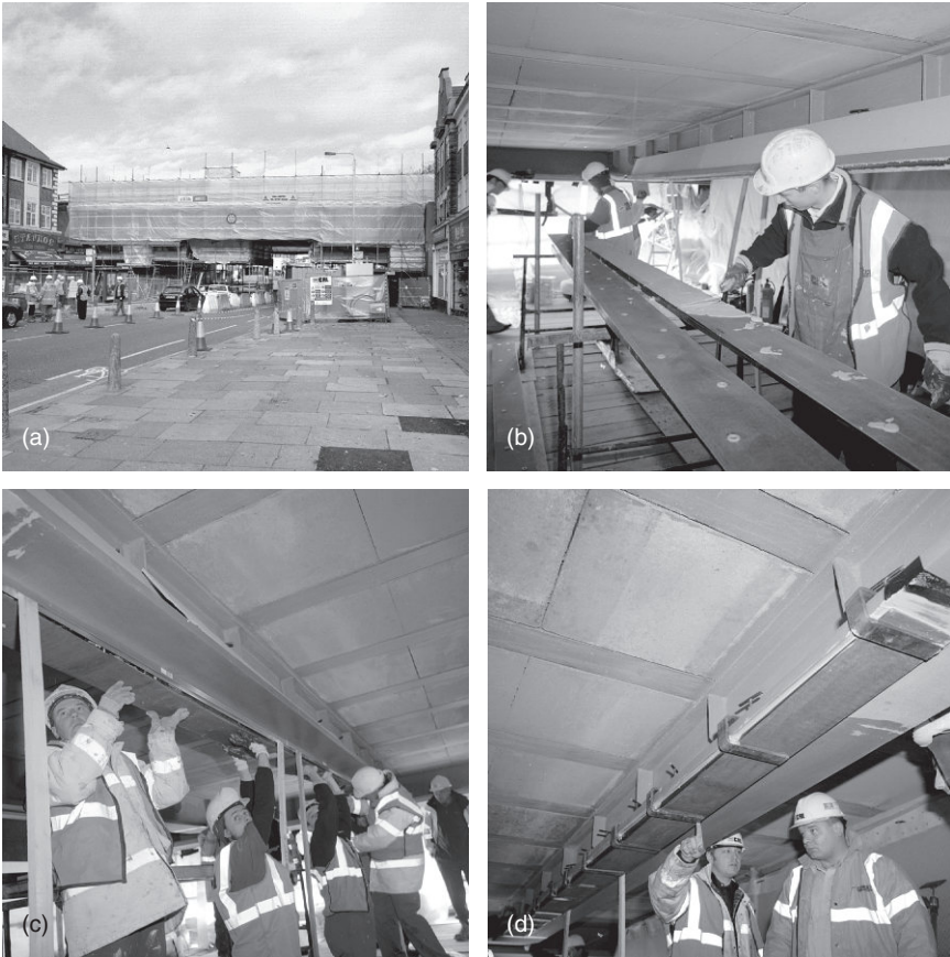
12.9 The various stages of upgrading bridge MR46A that carries twin rail tracks over Station Road, Harrow, adjacent to North Harrow Station (courtesy of Sika Ltd and CRL). (a) The bridge clad in polythene sheeting to give a weatherproof enclosure. (b) The adhesive being applied to the CFRP composite half plates. (c) The CFRP composite half plate being lifted into position. (d) The half plate being temporarily supported during the polymerisation of the adhesive. (This support is removed after about one week.)
