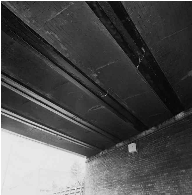
12.5 The upgrading of King Street Railway Bridge (courtesy of Tony Gee and Partners).
