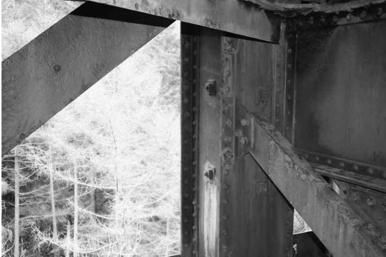
14.7 Wrought iron girders erected 1886 to replace a Brunel designed wooden viaduct, Largin, Cornwall, UK. Note general good condition.
