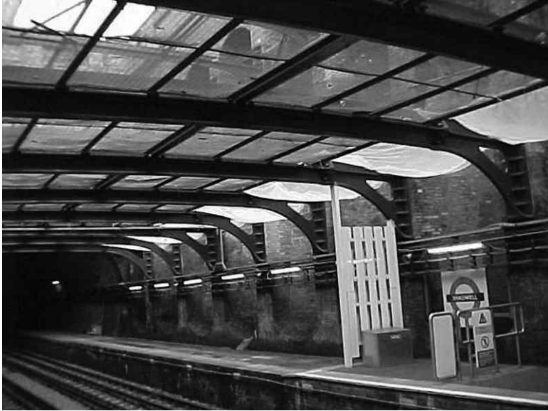
14.9 Cast iron struts at Shadwell Station, London Underground. Note upper and lower layers, cruciform section and elaborate end brackets.
