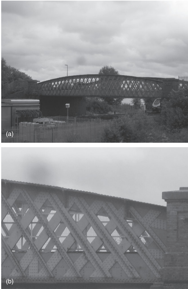
14.14 Horseshoe Bridge, Southampton, UK, a wrought iron truss bridge. Note the varying sizes of the diagonal members.
