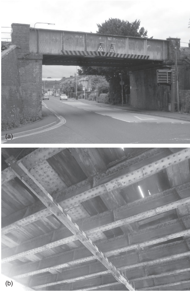
14.15 Views of a typical riveted wrought iron plate girder railway bridge, Romsey, Hampshire, UK.
