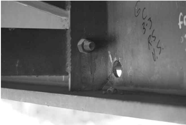
11.29 Fatigue crack in the bottom web-gap region of a steel bridge girder due to out-of-plane deformation induced by a cross-frame.
