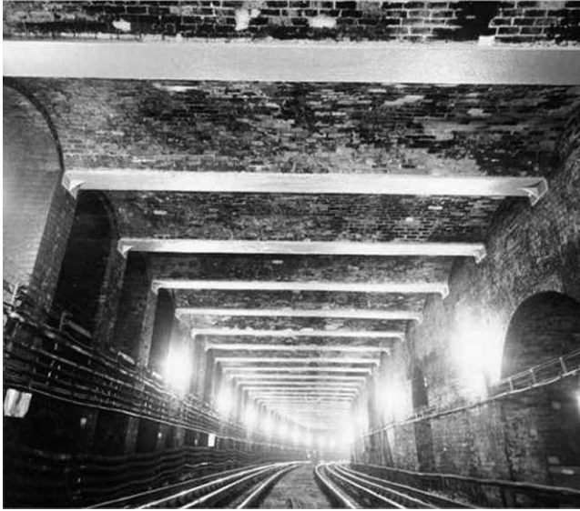
14.11 Cut and cover tunnel showing cast iron girders with brick arches between.
