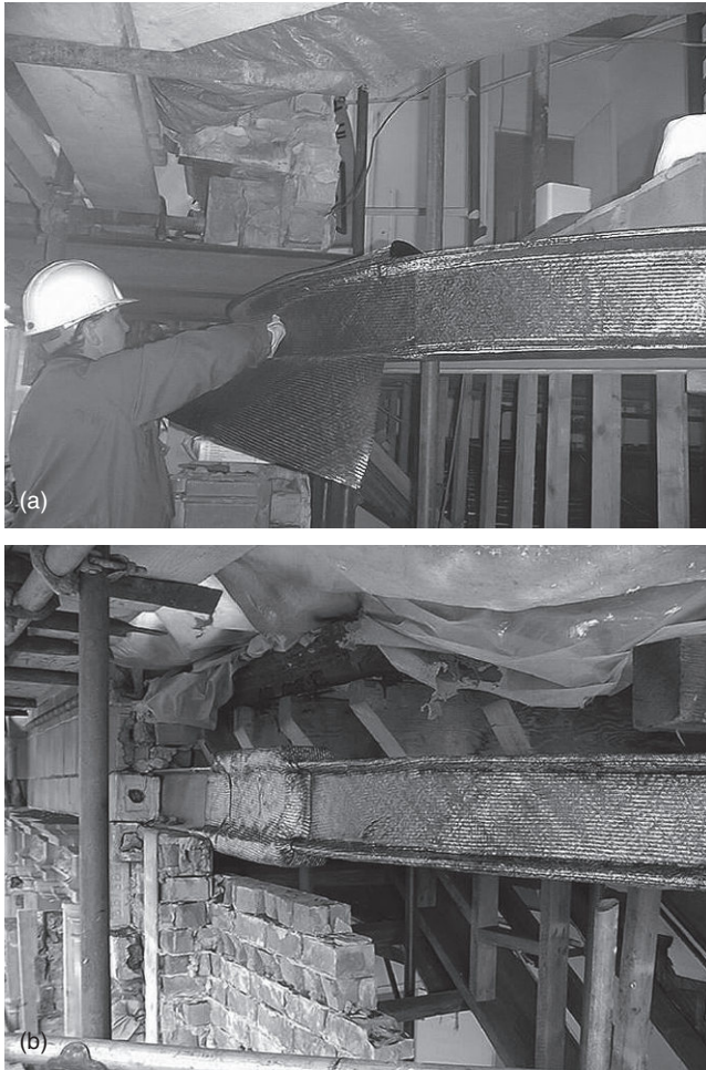
12.10 Strengthening the Boots Building, Nottingham: (a) final placement of the CFRP pre-preg around the flange and web of the aluminium beam; (b) CFRP pre-preg has been placed over the original bolted connections of the aluminium beam (courtesy of Vinci Construction, UK, and ACG, Derbyshire, UK). (First published in Hollaway and Cadei, 2002.)
