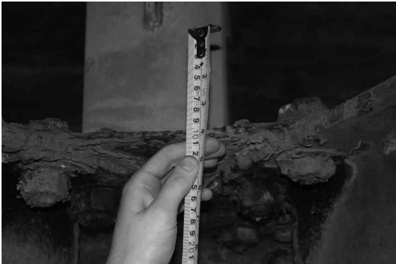
14.8 Heavy corrosion of wrought iron with delamination, also from Largin Viaduct, Cornwall, UK.
