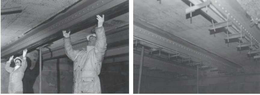
12.8 Installation and temporary clamping of CFRP plate at Slattocks Canal Bridge. (Courtesy of SKM, UK)
