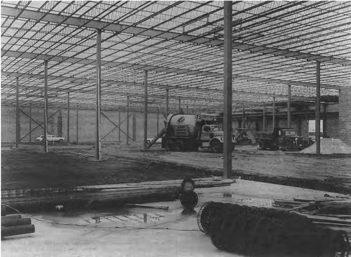
Fig. 12.1.10 A view of a plant during construction. Shown are its columns, roof trusses, and exterior masonry walls. The reinforced-concrete floor slab is being poured over compacted soil. (Source: VMA, Inc.)
