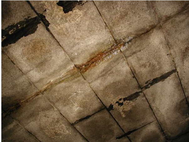
Fig. 9.24 Water leakage from the above before repairing.
