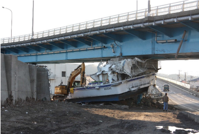
Fig. 2.6 Ship collision damage.
