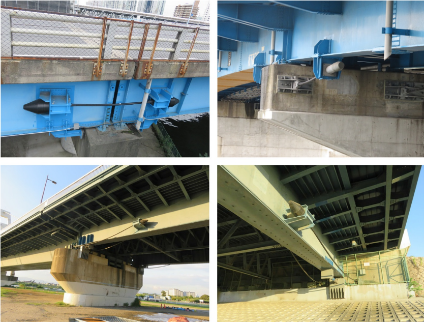
Fig. 5.7 Bridge fall preventing device. (Photos by Lin.)
