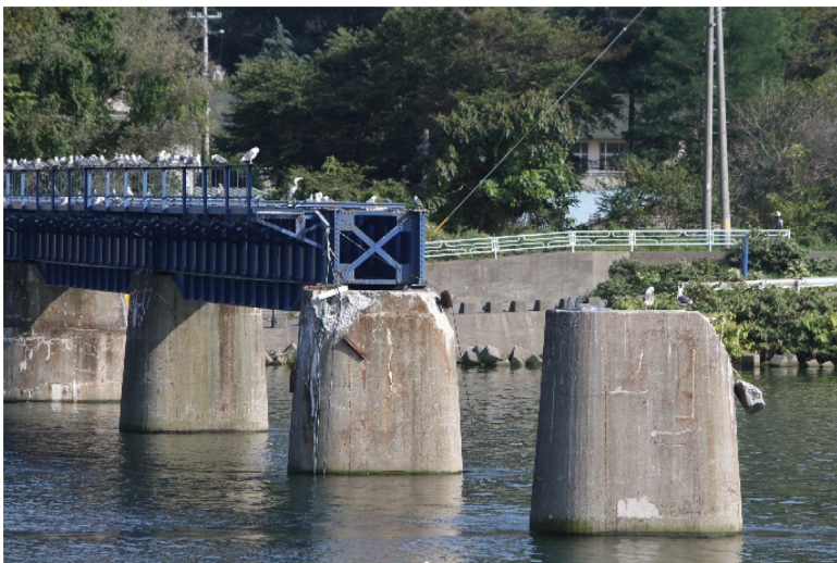
Fig. 2.5 Bridge partially swept away.
