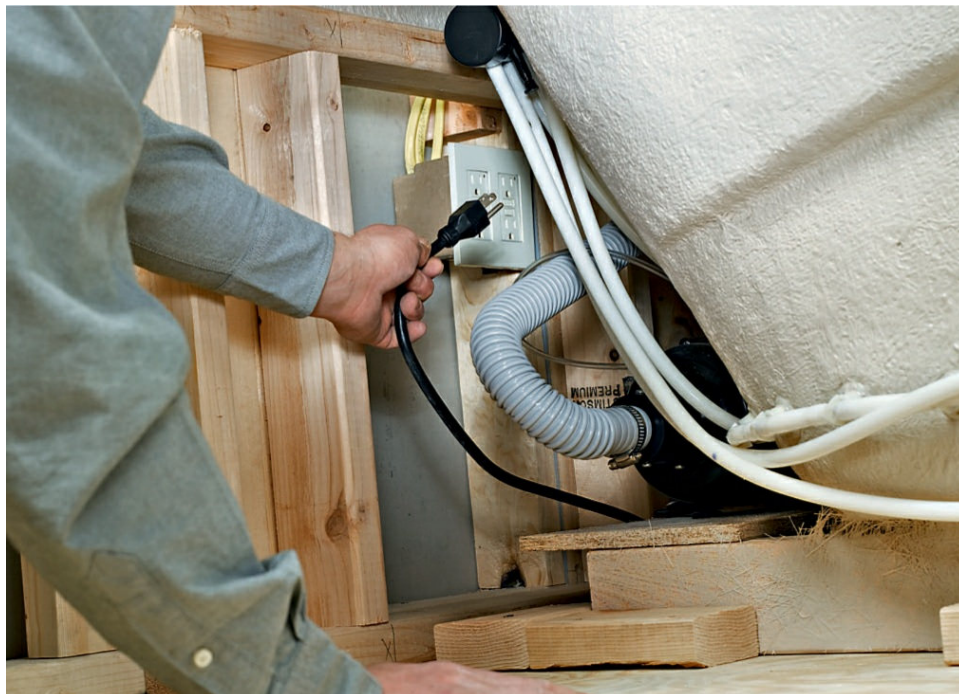
Receptacles for whirlpool tubs must be GFCI protected.
