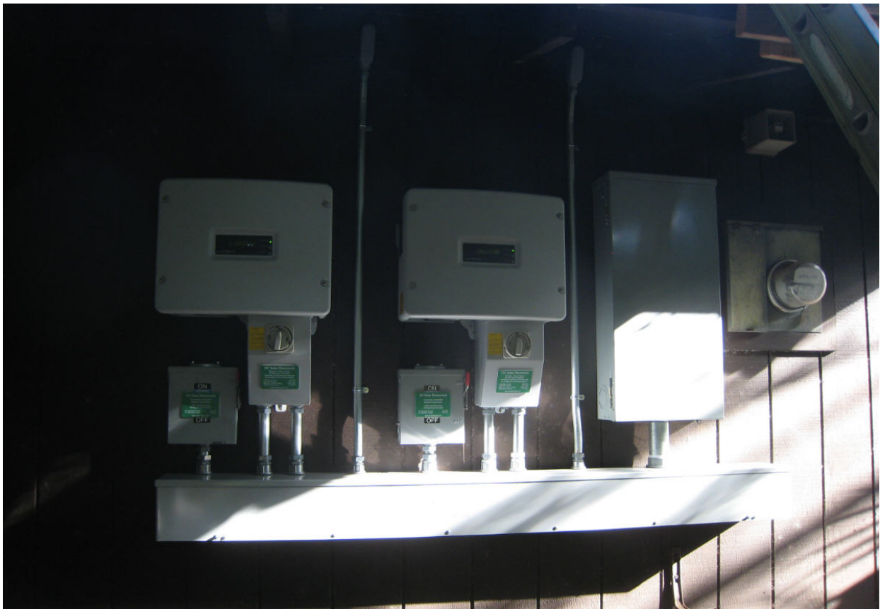
Figure 7-Multiple inverters with built in AC & DC Disconnects, gutter and 200 amp Sub Panel
