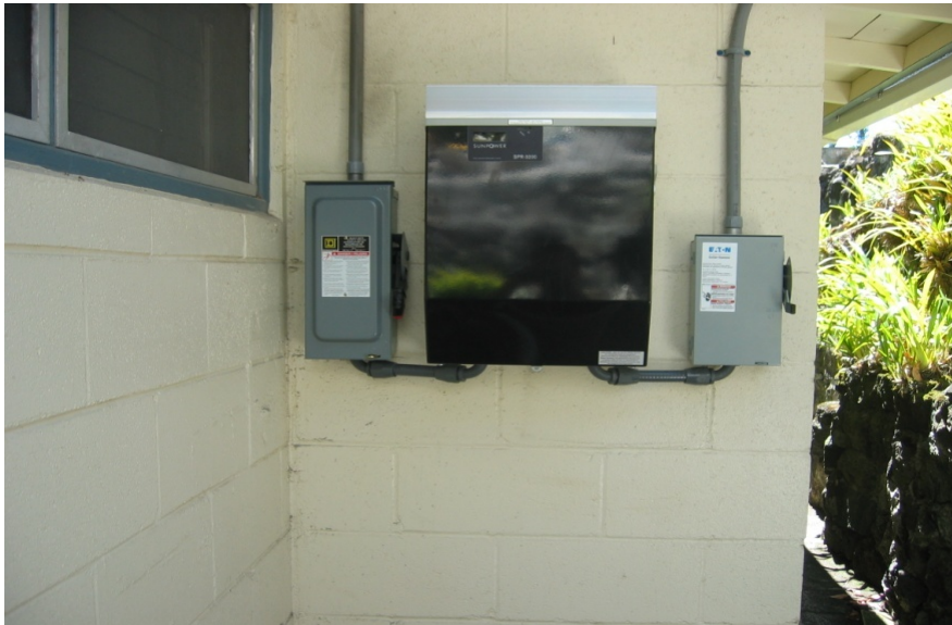
Figure 5-Single inverter with AC & DC disconnects as separate components
