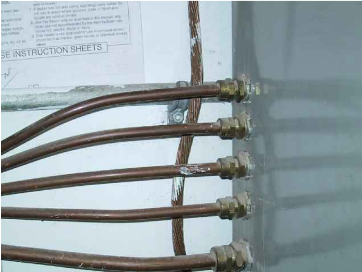
Mineral insulated cables at a panel board
