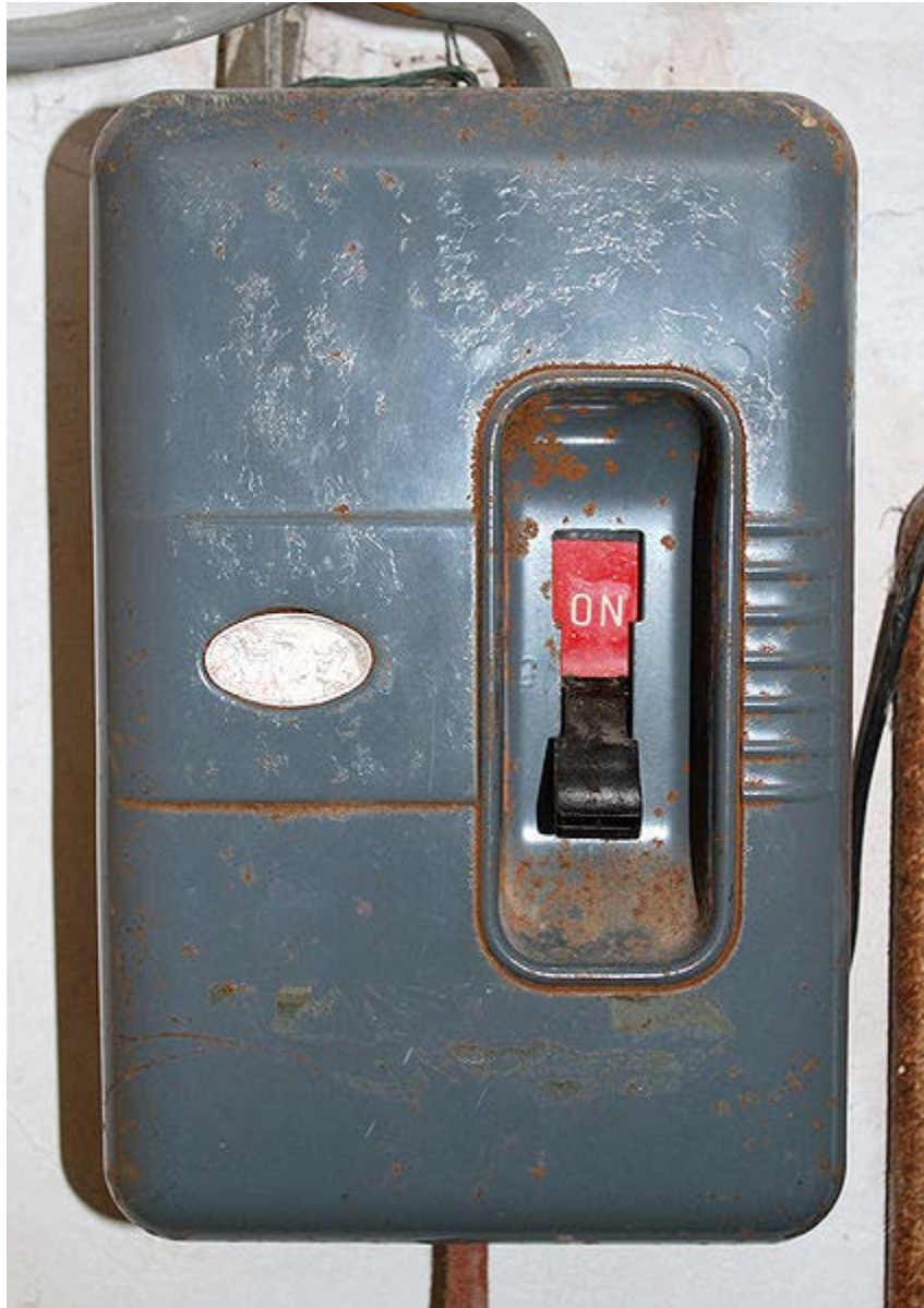
1950s MEM rewirable fuse box (covered)
