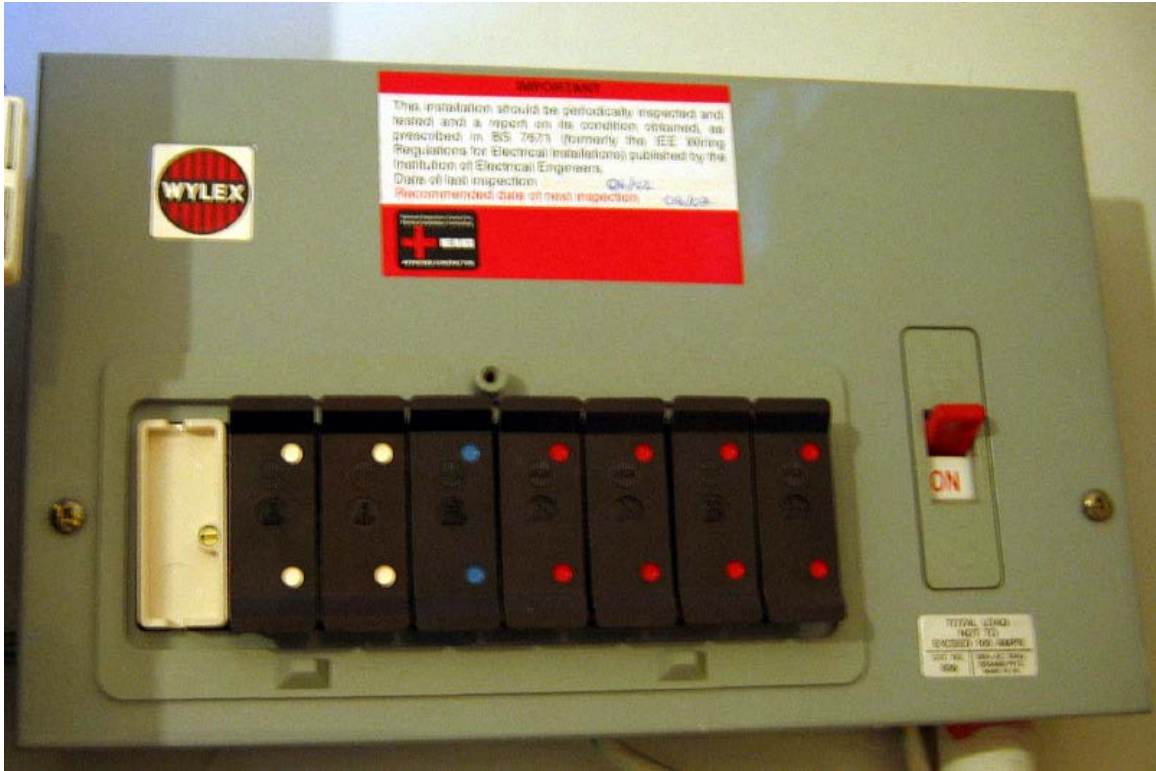
Wylex fuse box
