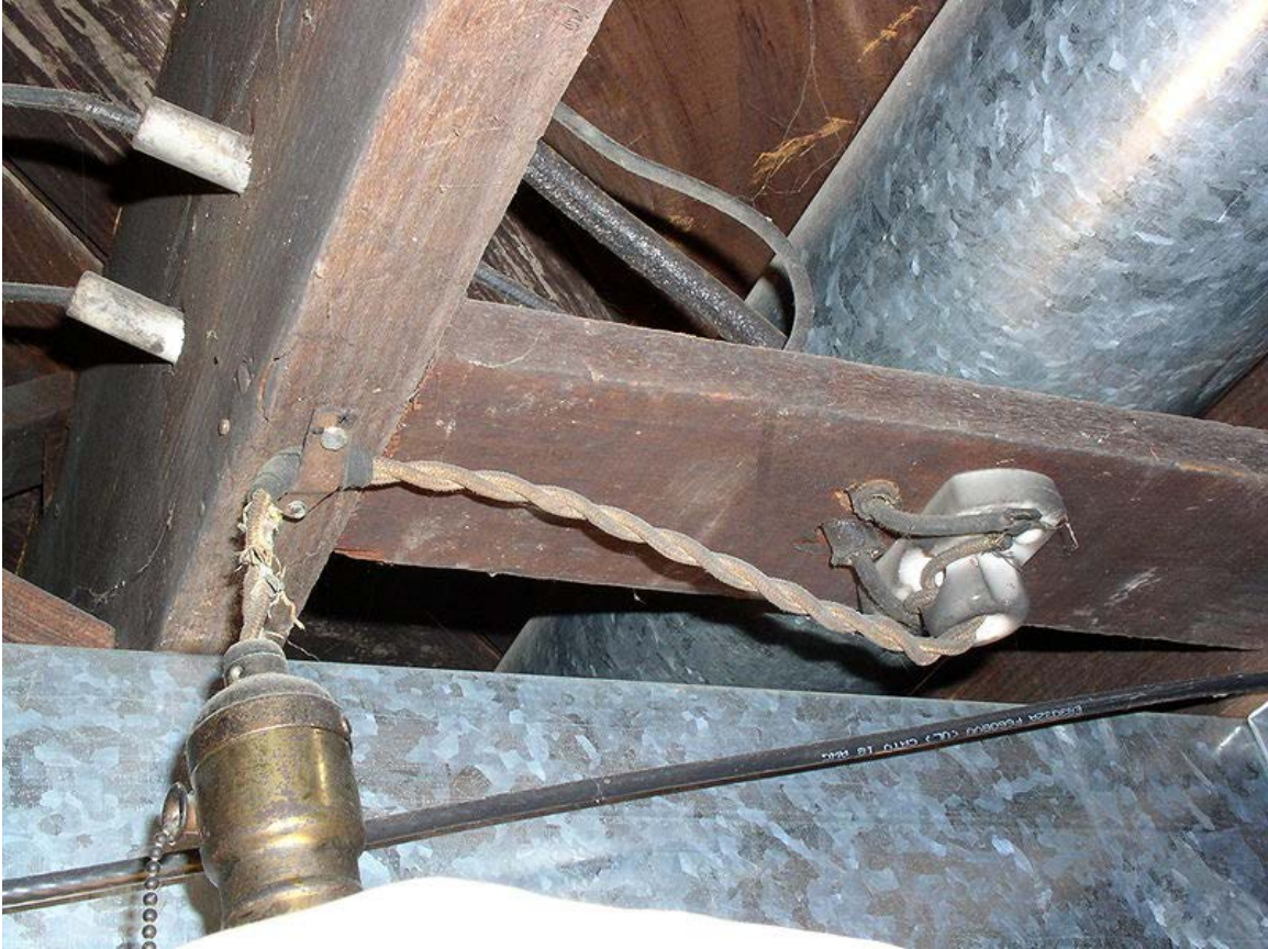
Ceramic junction for suspended light socket. Note deteriorated wire insulation.
