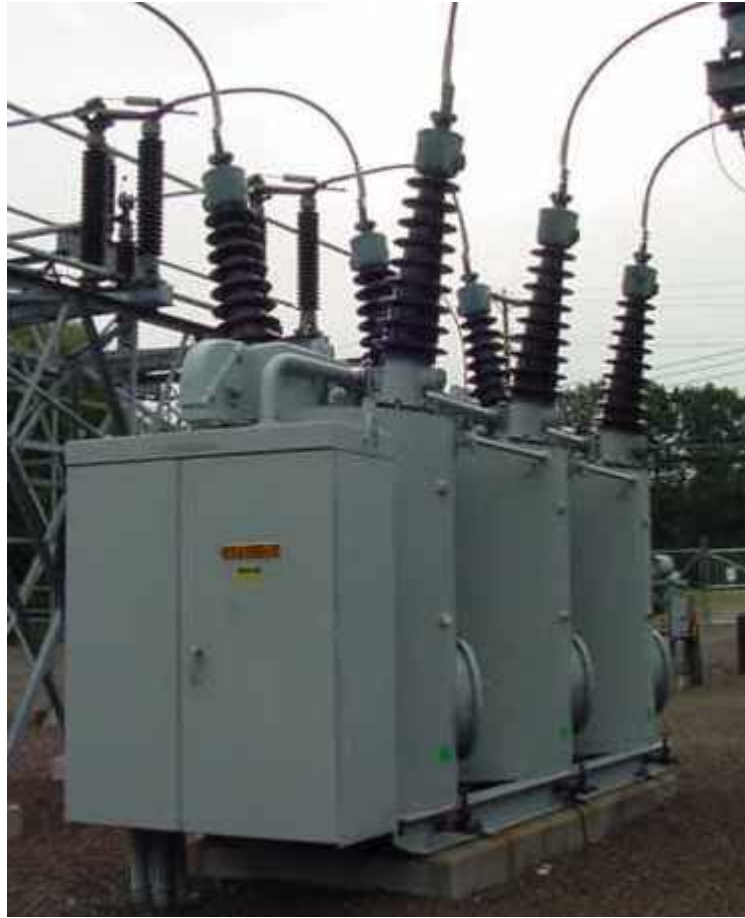
115 kV bulk oil circuit breaker
