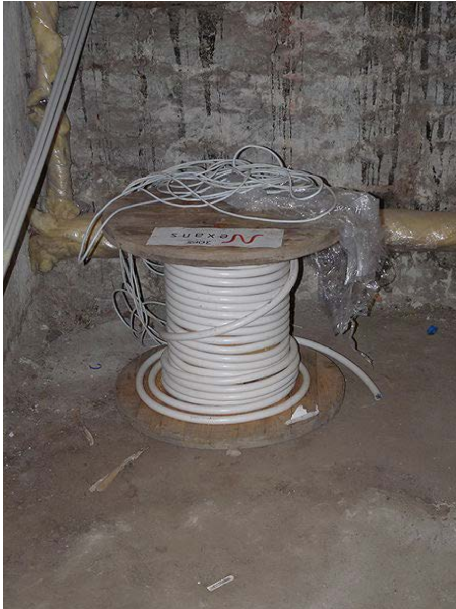
Three-phase copper cable TN-S 16mm 2 (5AWG) with PVC insulation
