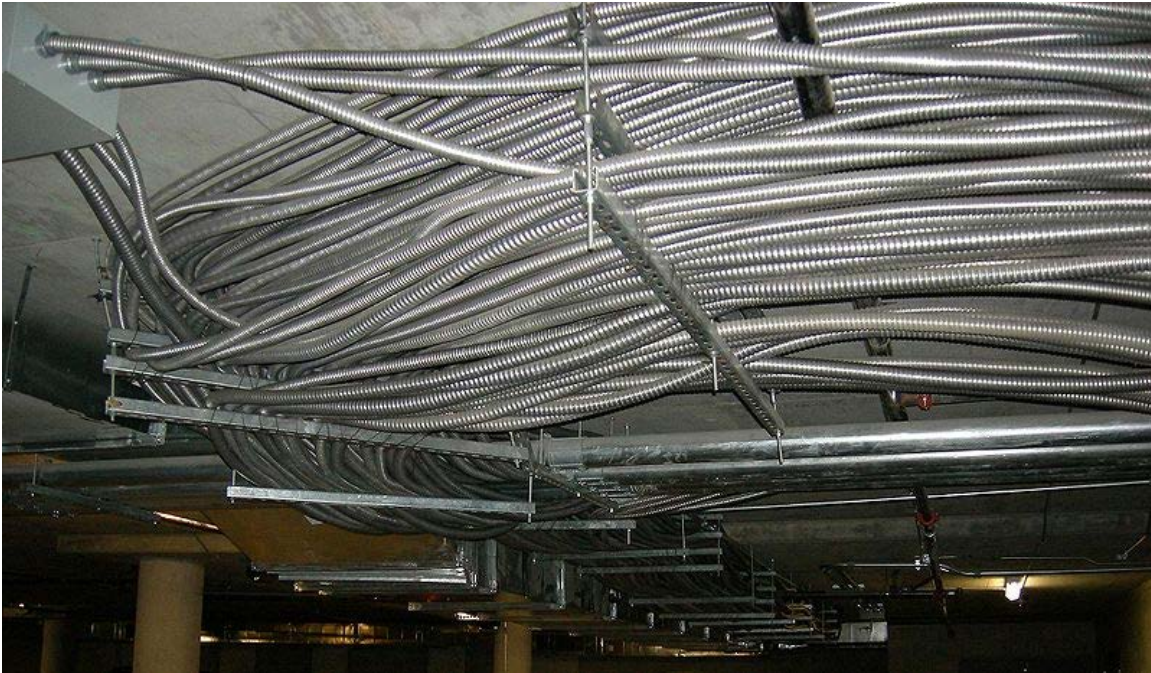
Flexible metallic conduit used in an underground parking facility.
