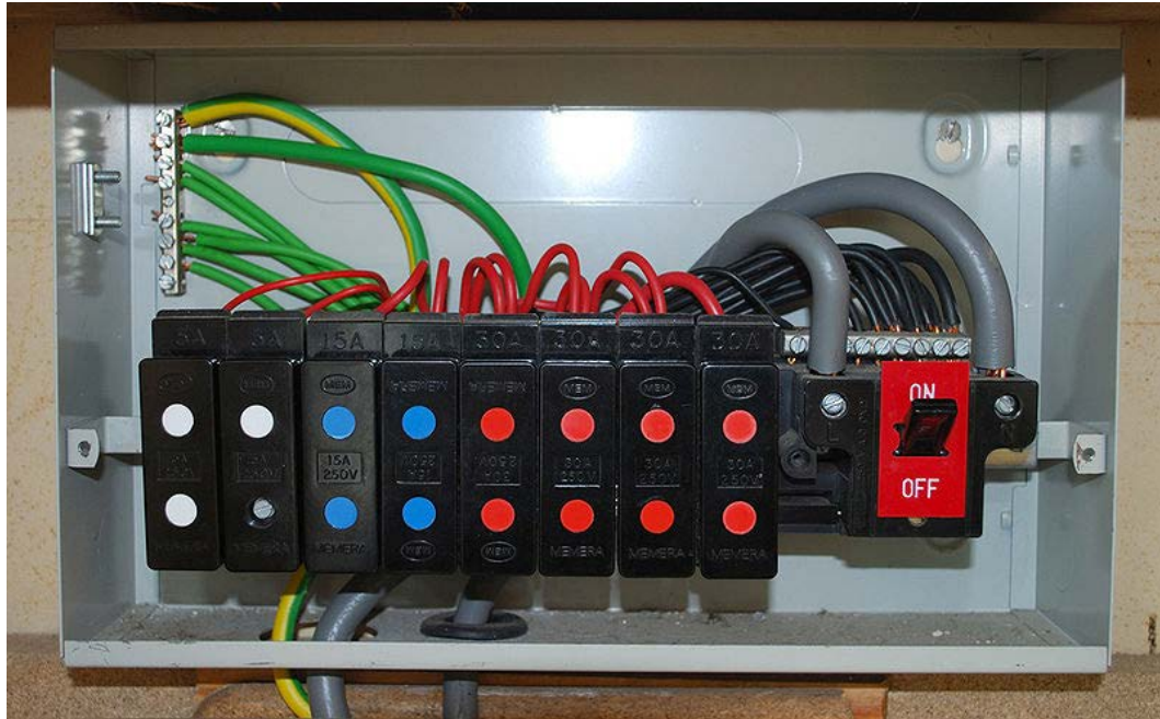
1970s MEM rewirable fuse box (open)
