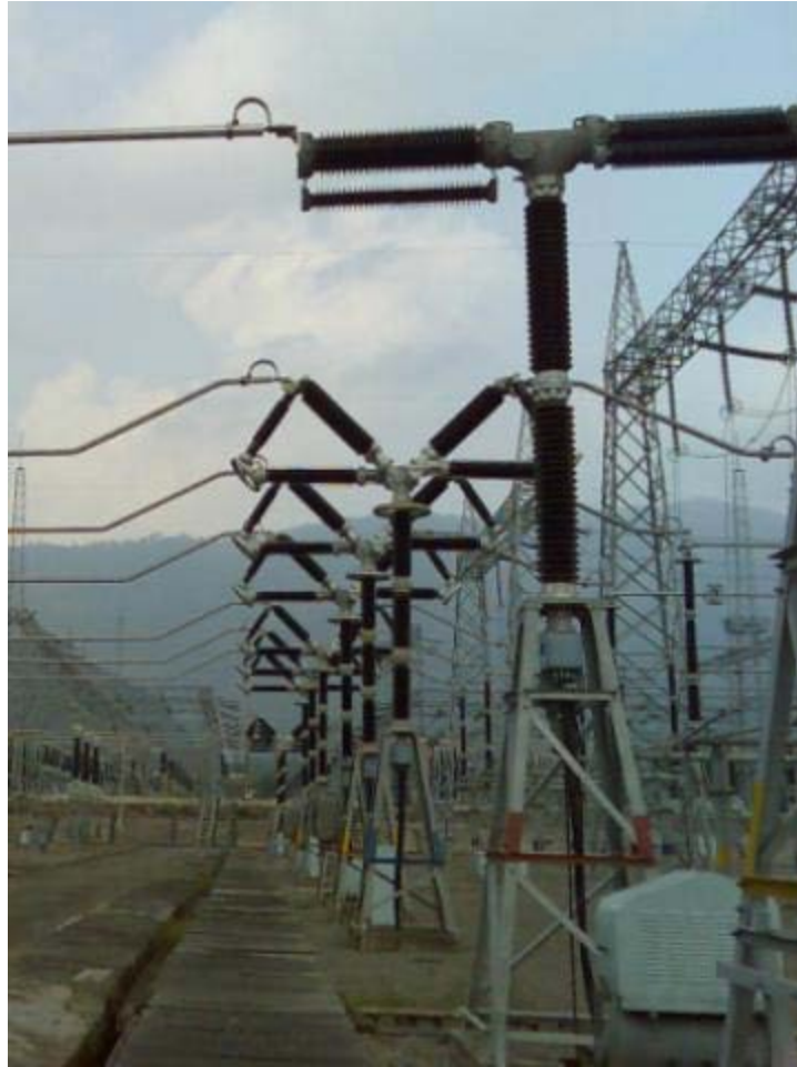
400 kV SF 6 live tank circuit breakers
