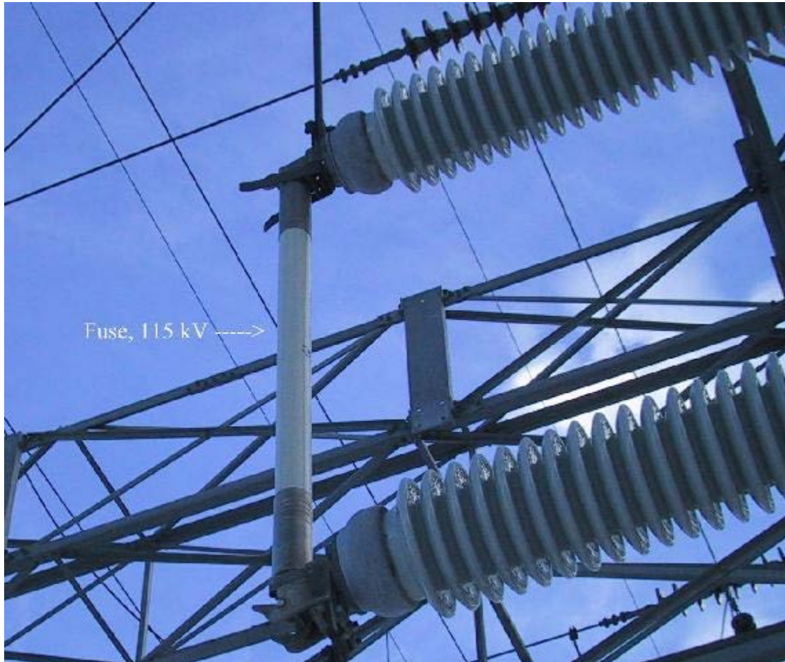
A 115 kV high-voltage fuse in a substation near a hydroelectric power plant.
