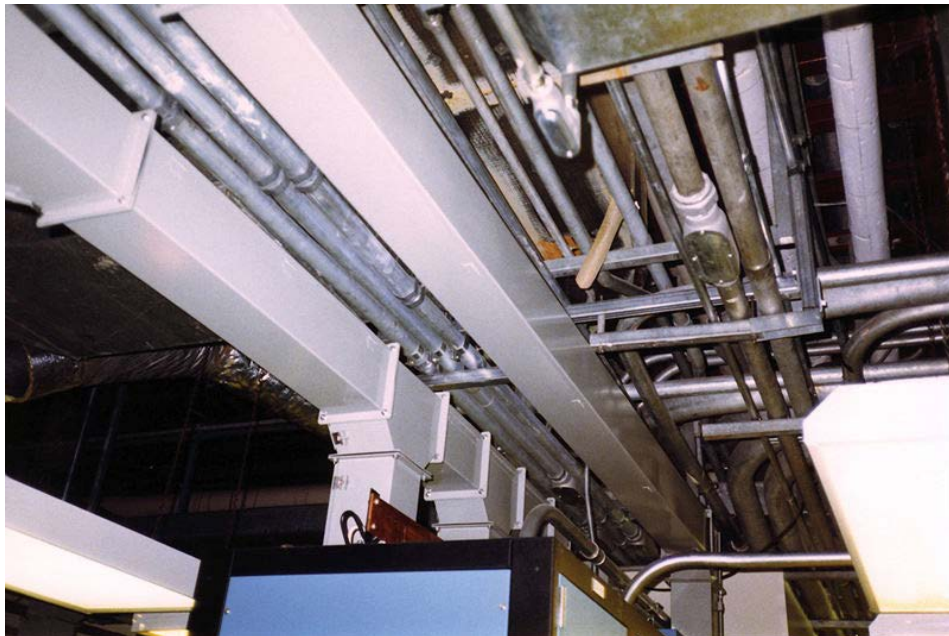
Electrical conduit and bus duct in a building at Texaco Nanticoke refinery in Nanticoke, Ontario, 1980s.
