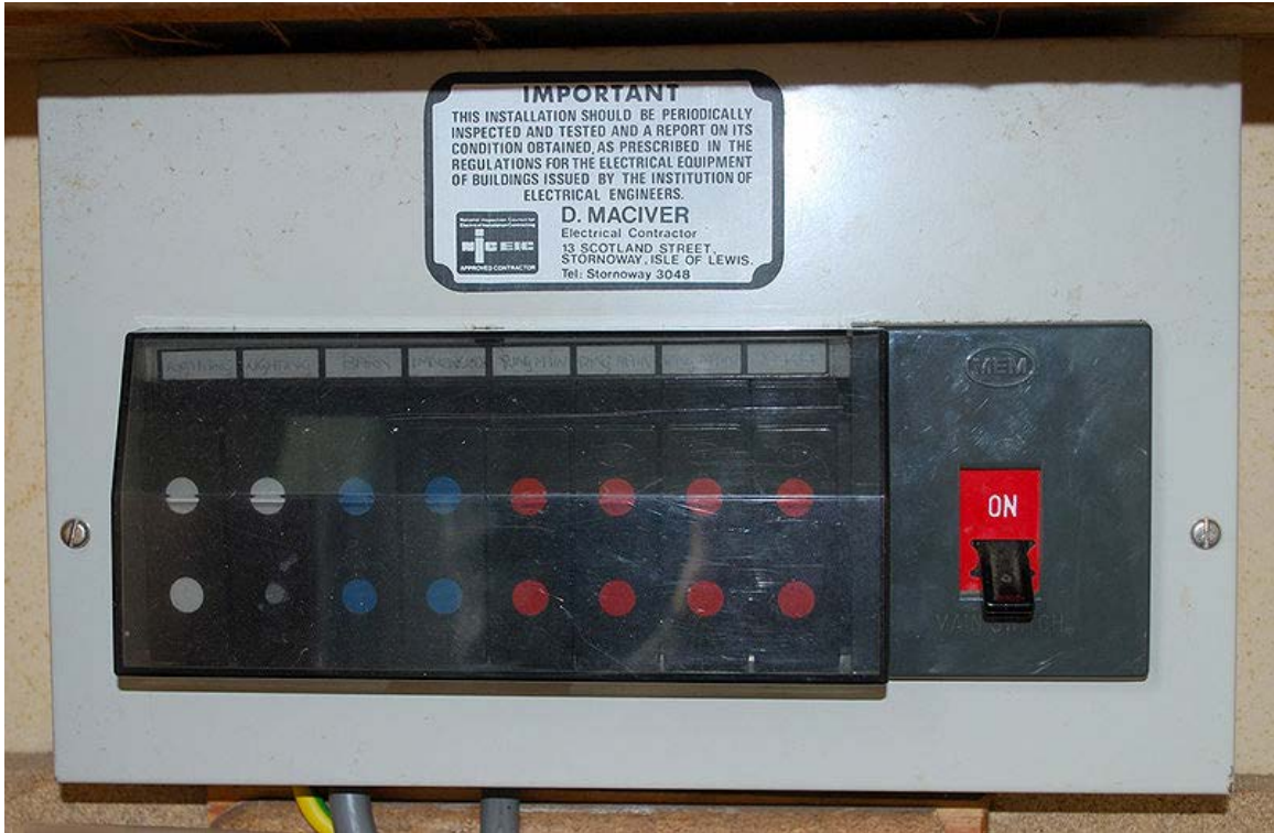
1970s MEM rewirable fuse box (covered)
