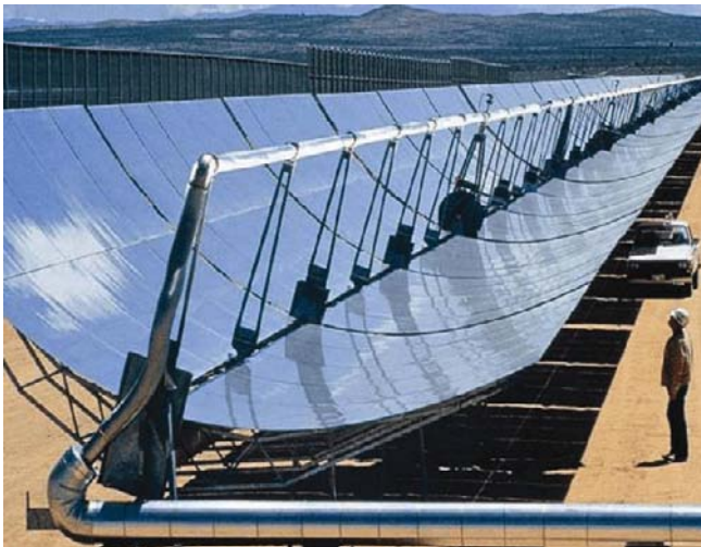
Figure 26. Representative Solar Thermal Plant: Nevada Solar One
