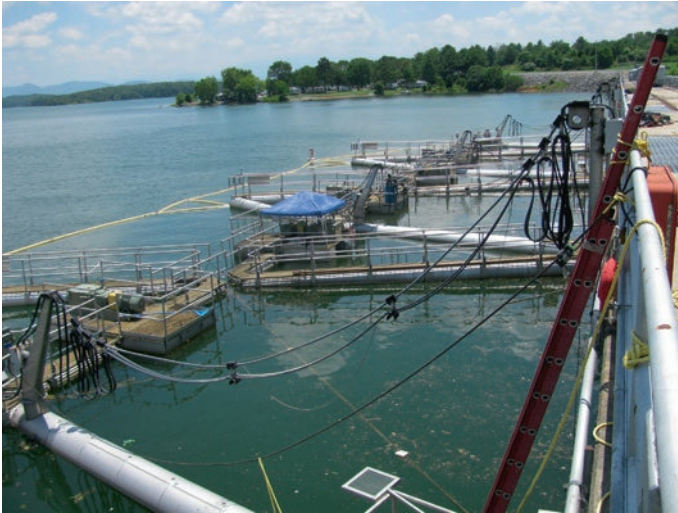
Fig. 13.3 Surface-water pumps help oxygenate the water in deeper reservoirs, resulting in improved dissolved oxygen concentrations downstream
