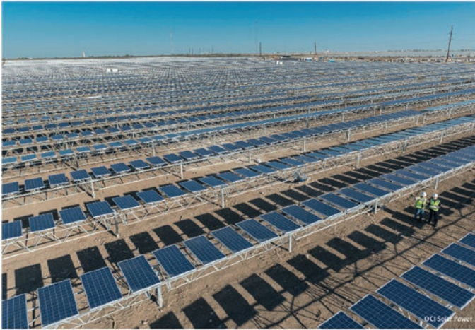
The Alamo 4 Solar Farm in Brackettville.
