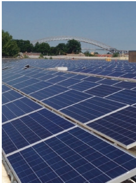
Fig. 4.4 View from the Port Richmond WWTP rooftop. Source Port Richmond Waste Water Treatment Plant Solar Array, New York. Personal photograph by author. 2014
