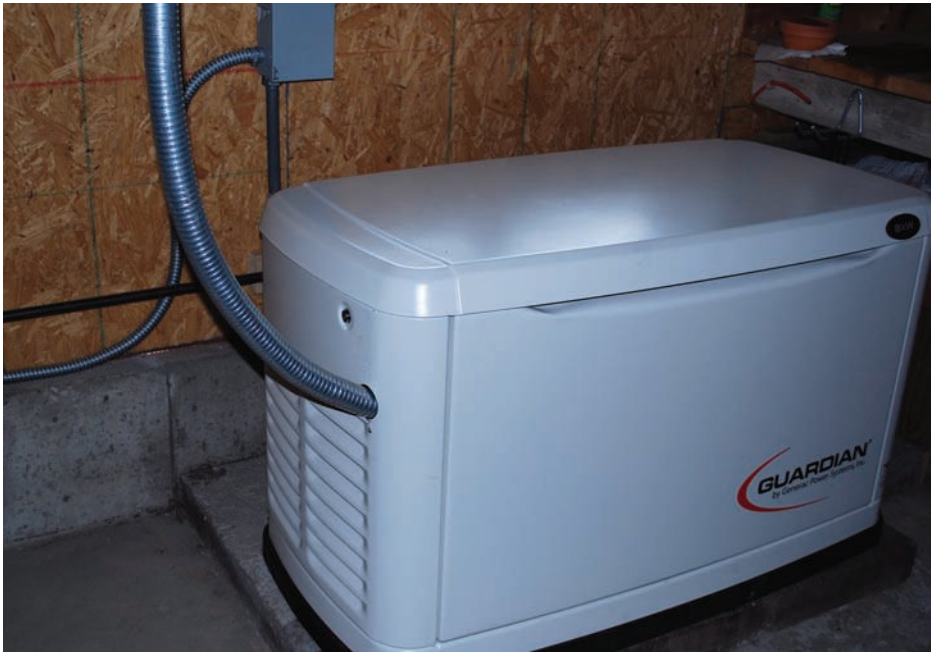
FIGURE 13-1 A small high-end generator.
