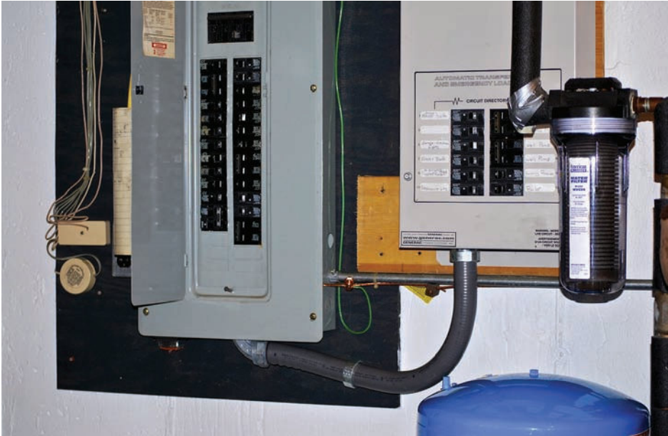
FIGURE 5-4 Note the clear violation of working-space requirements.
