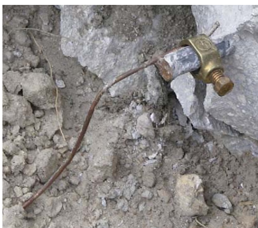
Figure 5.12 A bonding jumper attached to rebar which is encased in concrete.
