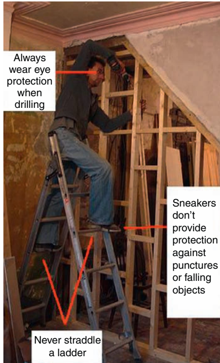
Figure 11.19 Three safety hazards by one worker.
