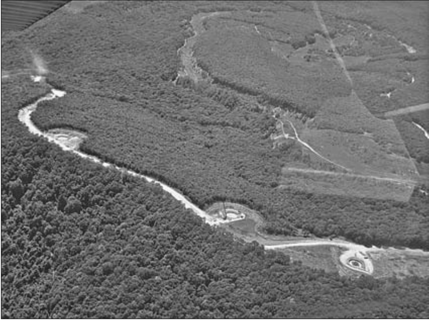
Partially constructed wind turbine sites line a ridgeline in Greenbrier County, West Virginia. Some of the sites will be decommissioned due to a federal court ruling. (Courtesy of Mountain Communities for Responsible Energy.)
