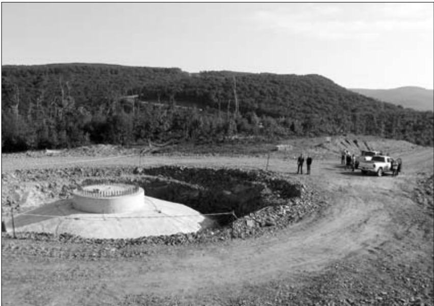
A wind turbine foundation under construction at the Beech Ridge site in West Virginia. (Courtesy of Mountain Communities for Responsible Energy.)
