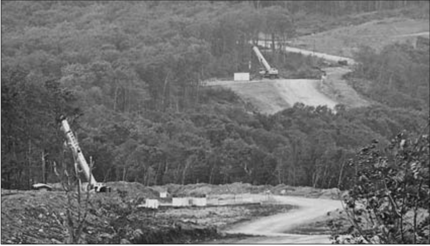
Construction begins on the Beech Ridge wind farm in Greenbrier County, West Virginia. (Courtesy of Mountain Communities for Responsible Energy.)
