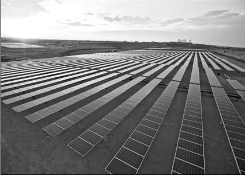
This solar cell (photovoltaic) installation is located at Denver International Airport. (Courtesy of the National Renewable Energy Laboratory.)
