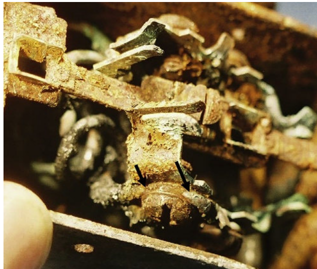
Figure 7.1: Glowing contact example – receptacle terminal screw
