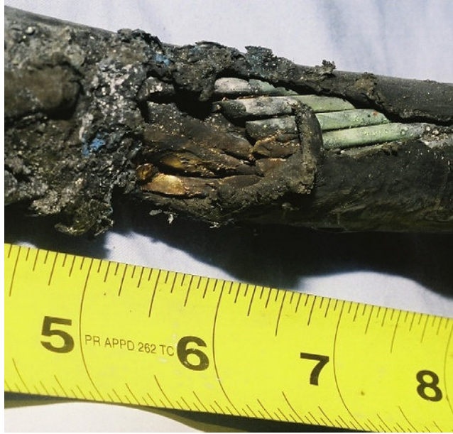
Figure 7.3: Wire insulation failure (from a fire) with resulting short circuit arc damage
