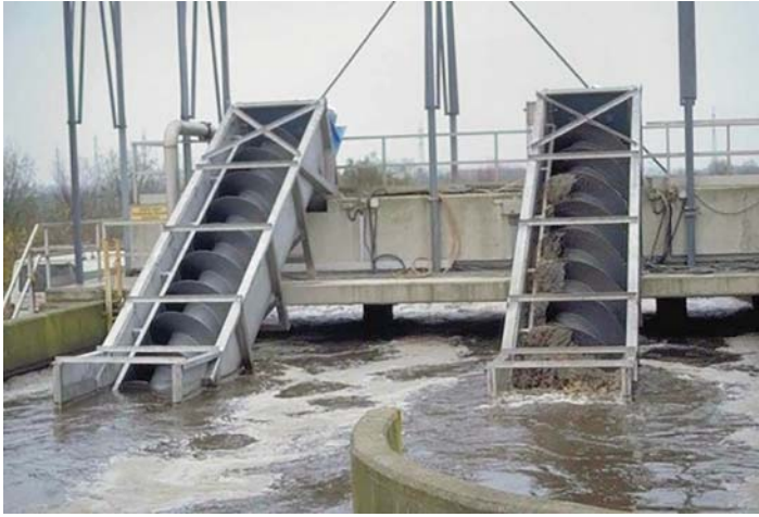
Figure 3.102 Archimedes screw on a site. Source: Dewekom Engineering.
