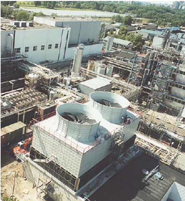
Figure 9.58 Cooling tower. Source: Howden.
