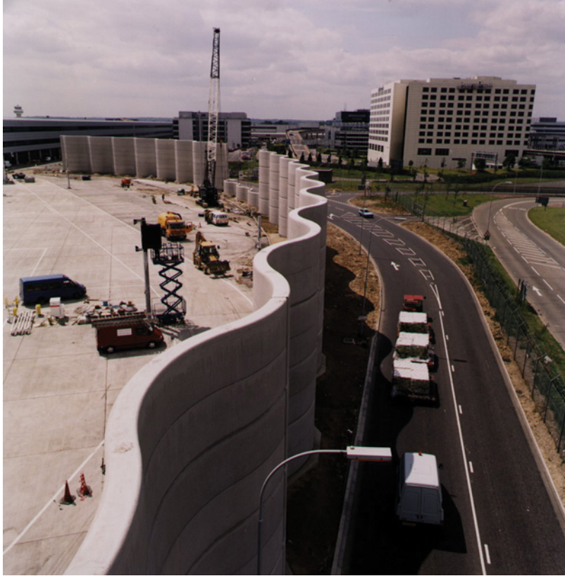
Figure 2.4 The wave wall at Gatwick contains noise from manoeuvring aircraft. Reproduced by permission of Buchan Concrete.
