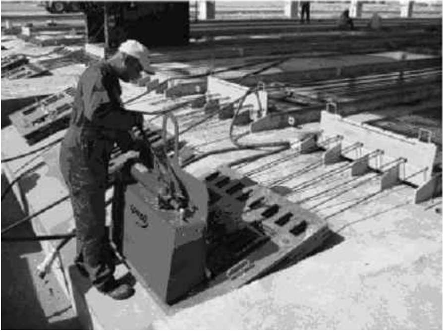
Fig. 2.2a Photograph of a pre-tensioning bed Photo courtesy of CCL
