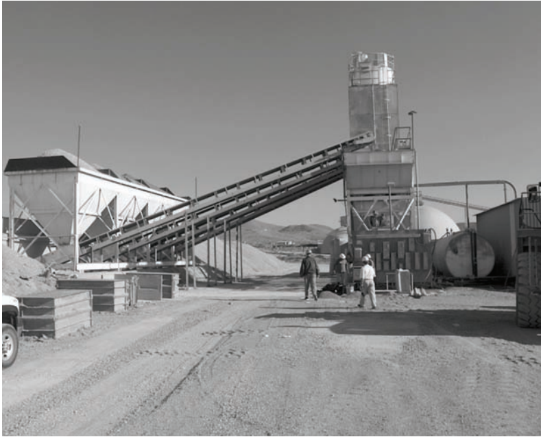
FIGURE 7.5 Concrete ready mix plant.
