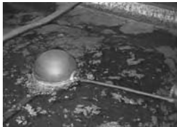
Figure 4.8 Galvanised tank corrosion
