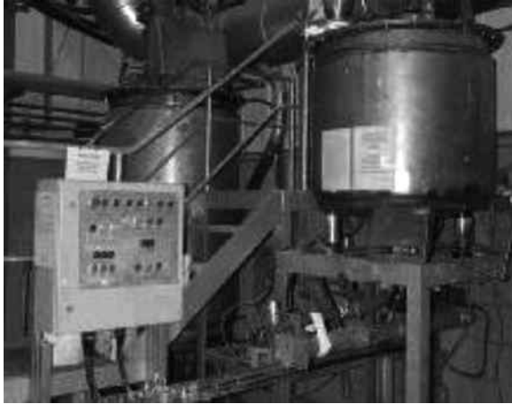
FIGURE 7.1 Mixing Vessel with a Control Panel (Courtesy of David Thomson.)
