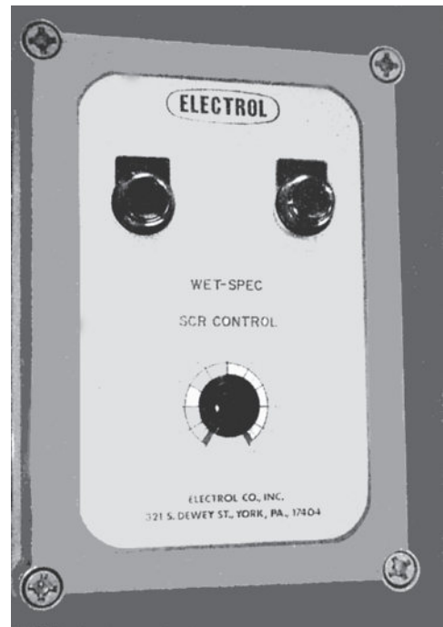
FIGURE 7-7 Control panel for SCR-controlled DC motor drive.
