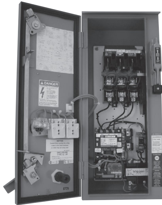
FIGURE 13–5 Combination starter with fusible disconnect switch.
