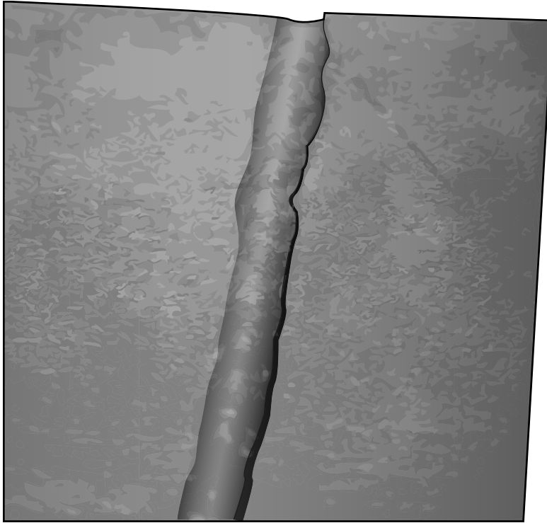
Figure 18-3: Example of a crack along a weld.
