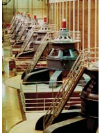
A series of hydral generators.
