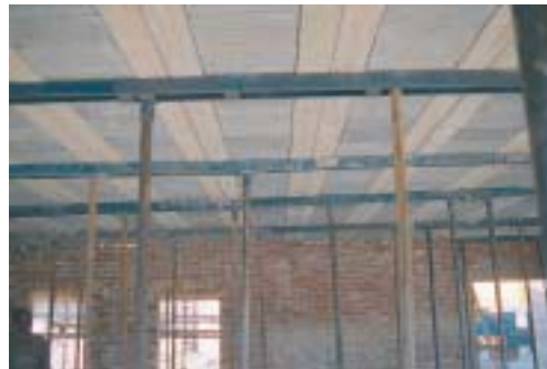
Figure 37: Propping under indicated positions.
