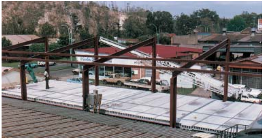
Figure 16: Hollow core slab on steel frame. Note omission of purlins for crane access.
