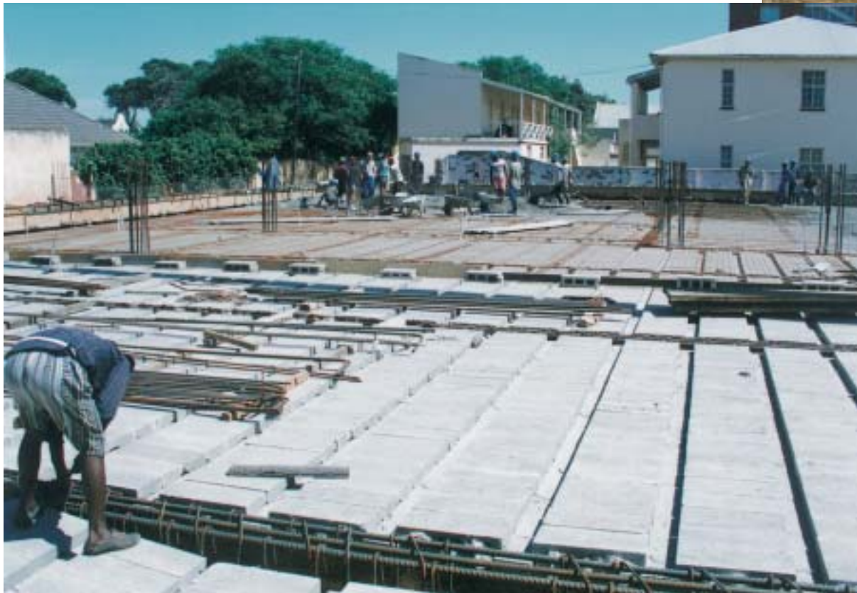
Figure 26: Preparing and casting of a precast beam and block slab in progress.
