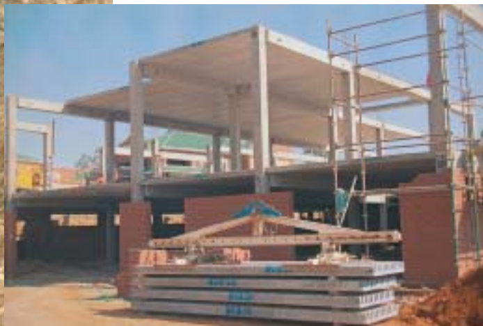
Figure 29: Precast hollow core slabs and precast beams erected on in situ columns.
