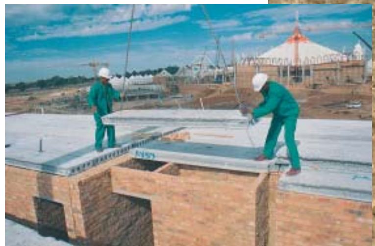
Figure 11: Hollow core slab being hoisted into position direct from the delivery vehicle by mobile crane.
