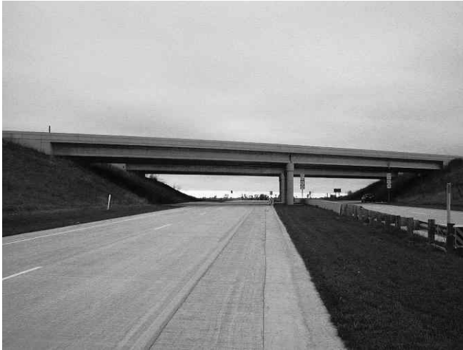
1.1 South side of US 151 overpass bridge, B-20-133. (Source: Courtesy of Dr Christopher Foley.)
