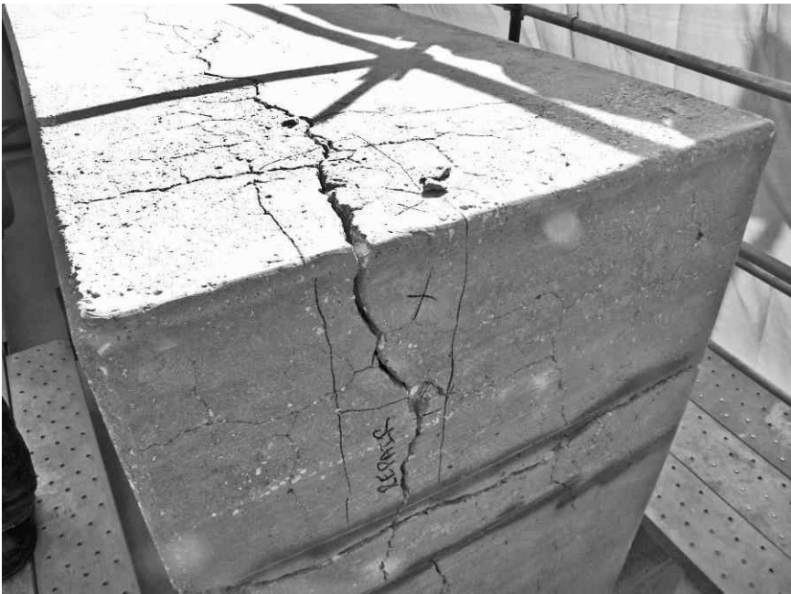
9.10 Severe cracking at end of straddle bent beam, prior to repair.
