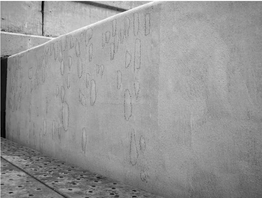
9.15 Areas of delamination marked after visual inspection of CFRP.
