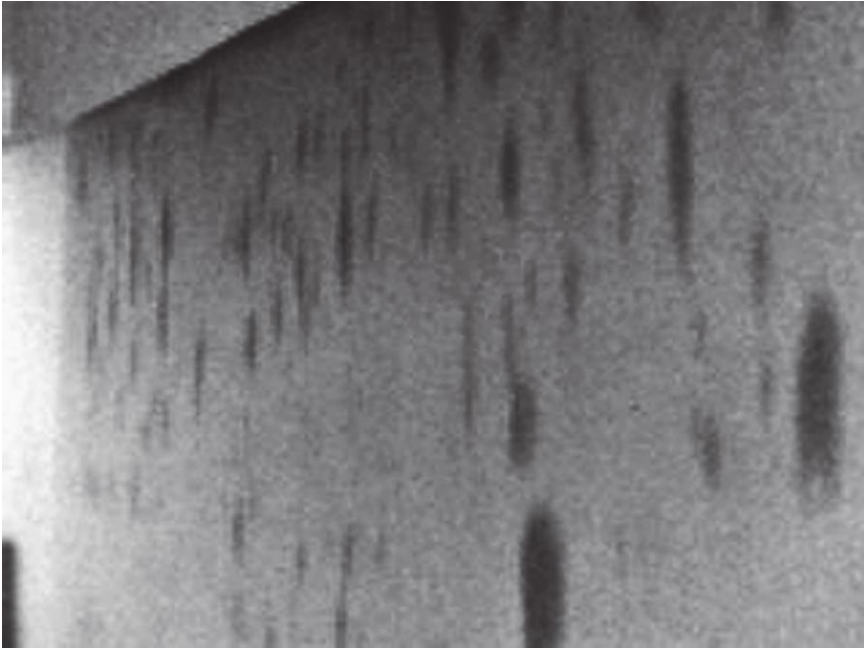
9.16 Areas of CFRP delamination identified by infrared thermography (black spots).
