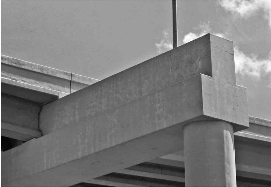
9.3 Partial elevation view of straddle bent with visible white staining exuding from cracks.
