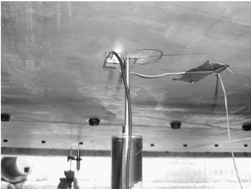
6.15 LVDT and accelerometer for the field testing in 2011.
