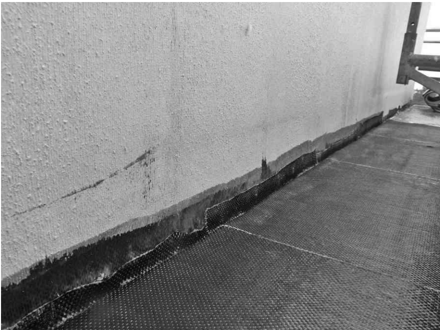
9.13 Application of CFRP composite anchor in slot (prior to final anchor installation).
