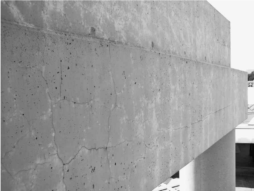
9.4 Map cracking with visible white staining exuding from cracks.
