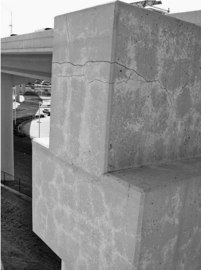
9.5 Severe cracking at end of straddle bent beam.
