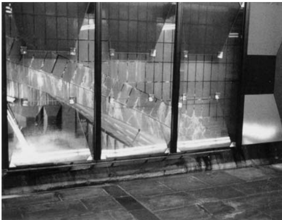
Figure 3.8.8 Leakages seen from the passenger bridge in the station.
