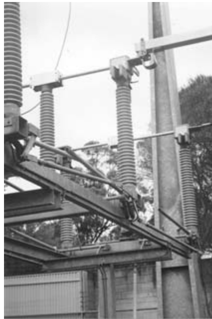
Figure 1.6 132 kV isolator with good corona design. Note automatic earthing arms in foreground
