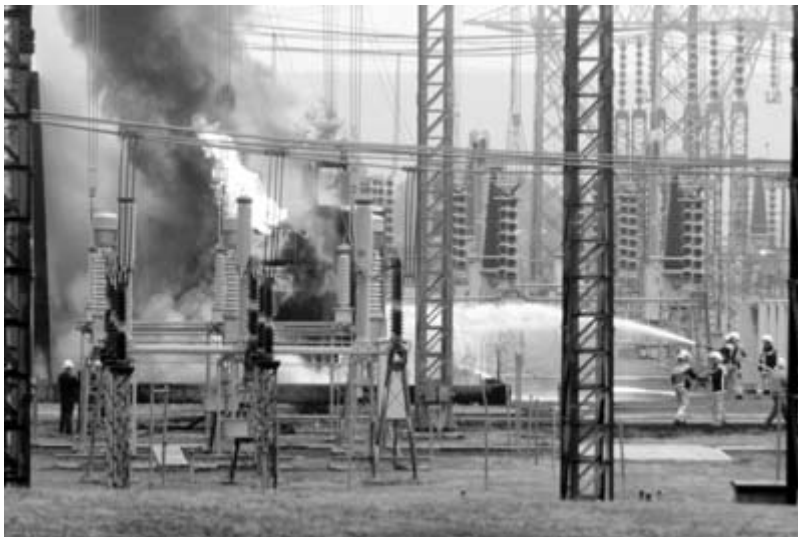
Figure 5.12 Fire following failure of a 330 kV transformer in a transmission substation [photograph by Brendan Esposito/Sydney Morning Herald]
