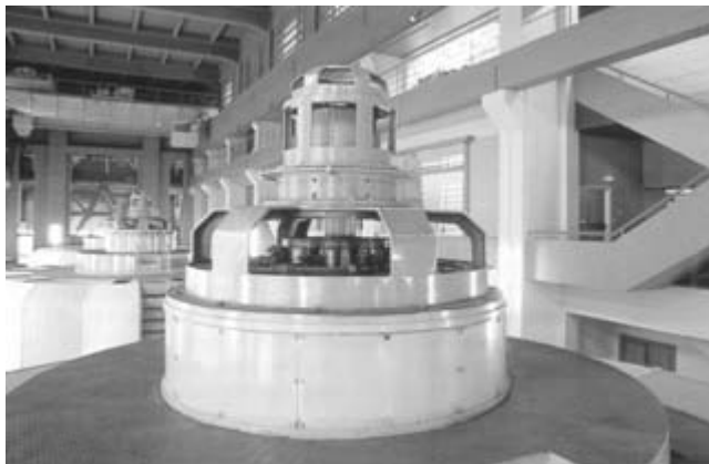
Figure 1.3 Hydro-generator [5] [reproduced by permission of CIGRE]
