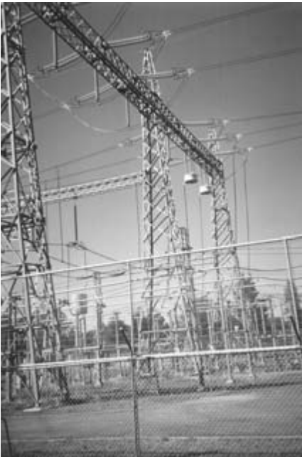
Figure 1.5 330 kV substation. Note insulator strings and corona rings [reproduced by permission of TRANSGRID, New South Wales]
