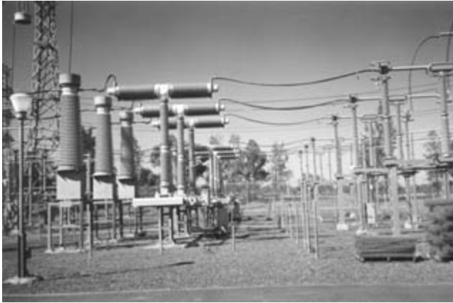
Figure 1.4 330 kV substation. Note (from left to right) – current transformers, SF 6 circuit breakers, support insulators for air isolators/automatic earthing arms [reproduced by permission of TRANSGRID, New South Wales]
