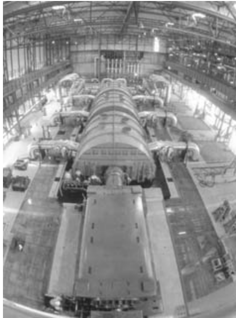
Figure 1.2 Steam turbine-generator [4] [reproduced by permission of CIGRE]
