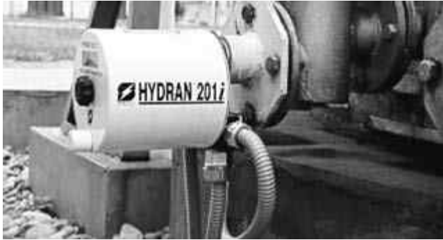
Figure 9.14 Online hydrogen monitoring on a transformer [13] [courtesy of GE Oil & Gas, http://www.gepower.com/prod_serv/products/substation_md/en/monitoring_instr_sys/hydran.htm ]
