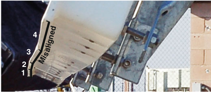
Fig. 12 Bottom-right view of misaligned HCPV modules
