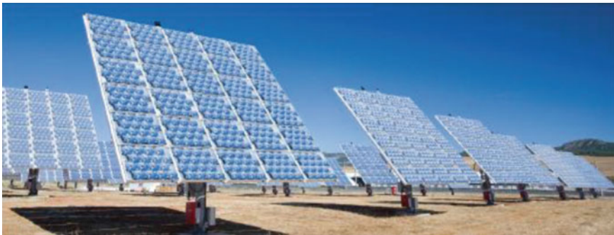
Fig. 22 Solfocus/ISFOC HCPV power plant ( courtesy of Solfocus/ISFOC)
