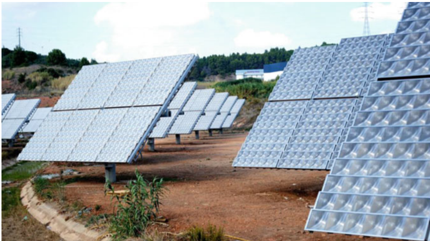
Fig. 23 Magpower HCPV power plant (courtesy of MagPower)
