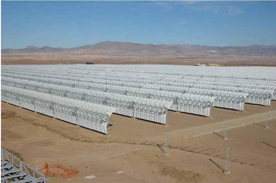
Fig. 2.15 Solar field of the Andasol-1 plant
