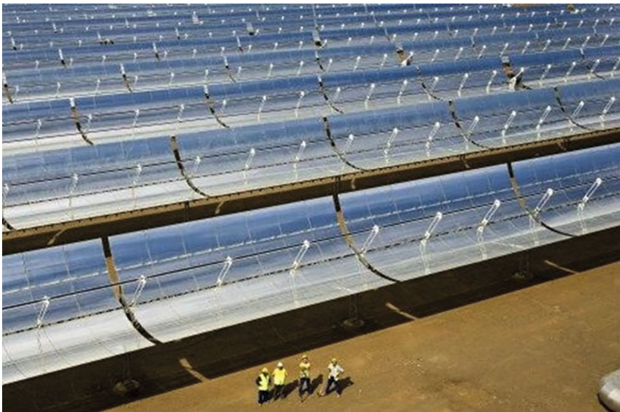
Fig. 4.6 Typical parabolic-trough collector solar field
