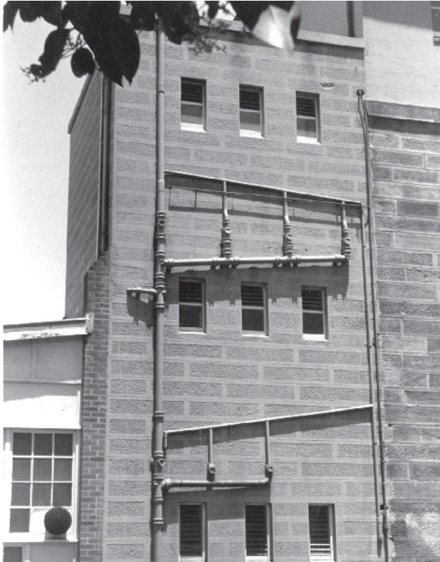
Cast iron pipes here showing externally for waste water drainage are easily identified by the heavy collars at joints.
