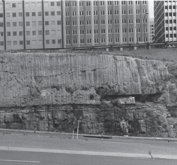
Cavities in apparently solid rock can be encountered in excavation.
