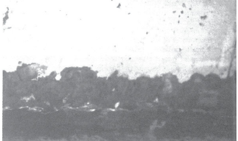
Deep staining of sandstone from rusting wrought iron fence post.
