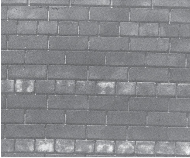
Efflorescence in header courses of a brick retaining wall due to salts conveyed from soil by water.
