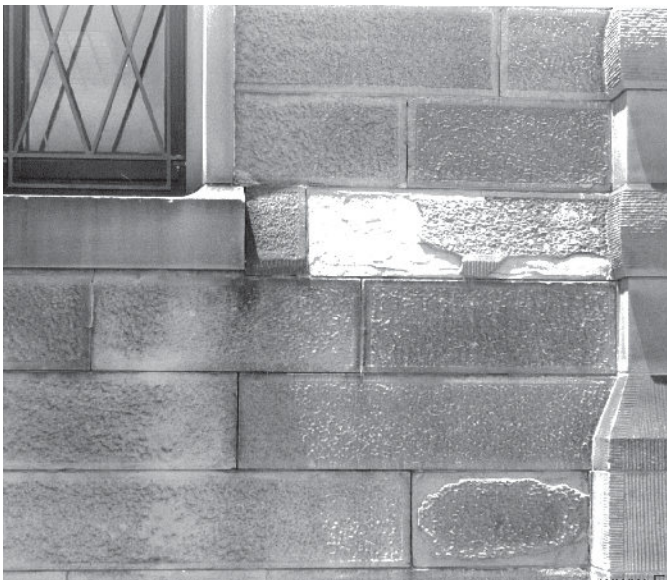
Fine jointed ashlar masonry showing differing deterioration of sandstone in adjacent blocks.
