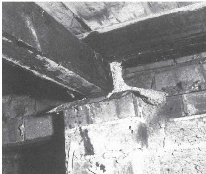
A termite access tunnel constructed to bypass a metal antcap and reach structural timbers.
