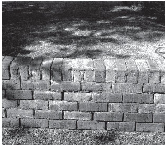
A 20-year-old fence of porous bricks badly affected by salty marine atmosphere.
