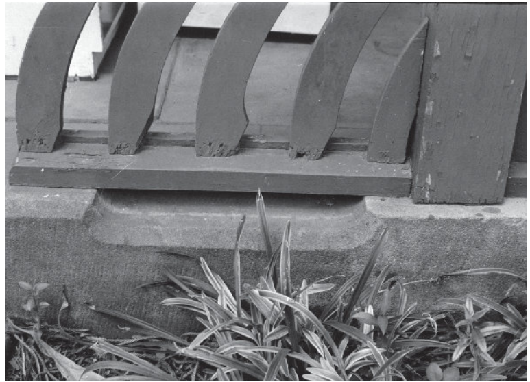
External timberwork showing signs of deterioration at joints due to weather exposure and insufficient maintenance of paintwork.
