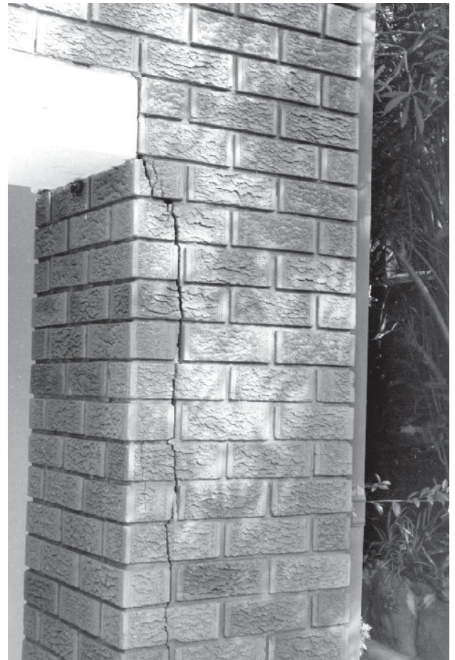
Brickwork cracking vertically near corner due to brick growth in long straight return wall.
