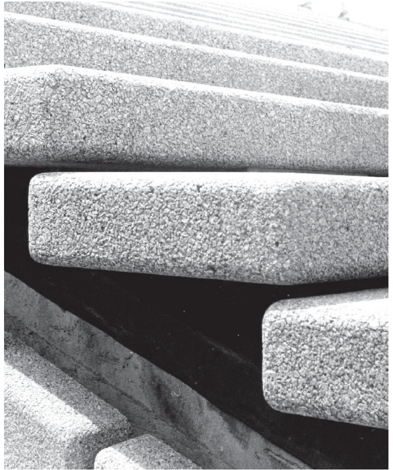
Reconstructed pink granite steps at Sydney Opera House - when over ten years old.
