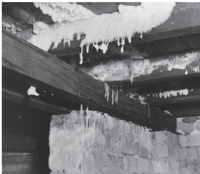
Floorboards and framing showing clear evidence of dry rot, a form of decay due to fungus.
