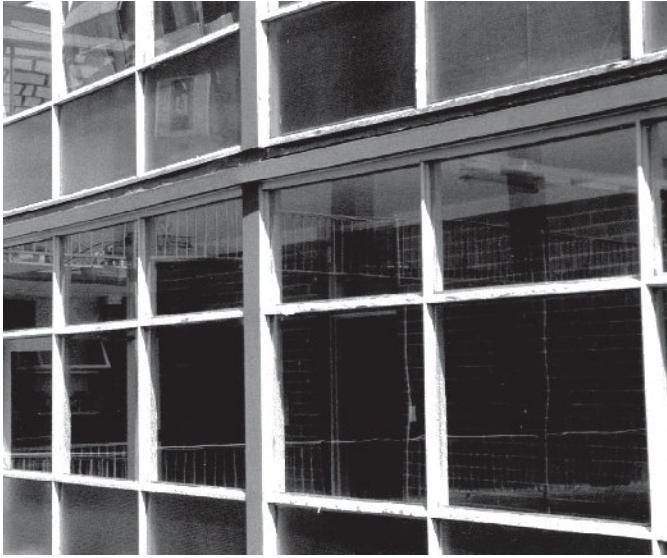
Gloss painted timber members showing two degrees of paint deterioration due to a 10-degree variation in the angle of exposure to the sun. The nearer timbers receive marginally more sunlight than the farther ones and show considerably more deterioration.
