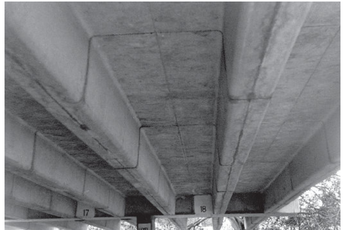
Joints in forms are often clearly visible in the concrete when stripped.
