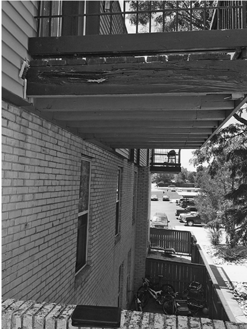
Figure 4.6 A common woodframe balcony showing signs of disrepair. (Image from “Cantilevered Balcony Safety” by Andy Engel, Fine Homebuilding, August 6, 2015.)
