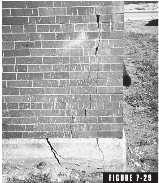
FIGURE 7-29 Cracking at building corner due to brick expansion restrained by concrete shrinkage.
