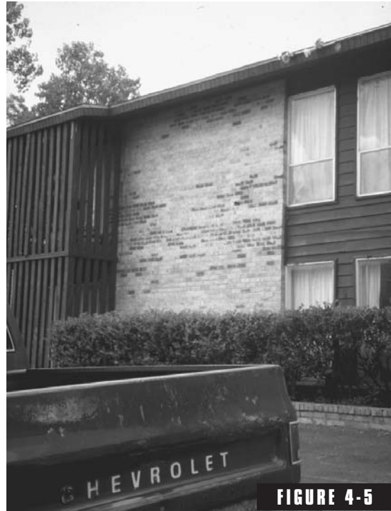
Figure 4-5 Uneven color distribution. (from Beall, Christine, Masonry Design and Detailing, 4th edition, McGraw-Hill, New York ).
