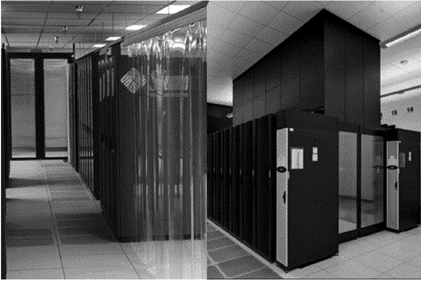
FIGURE 1.4 The picture on the left shows plastic curtains data centers have implemented to contain hot and cold temperatures. The picture on the right is a more viable solution but at an exponentially higher cost.
