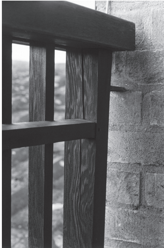
An 18-inch crack in another balustrade.
