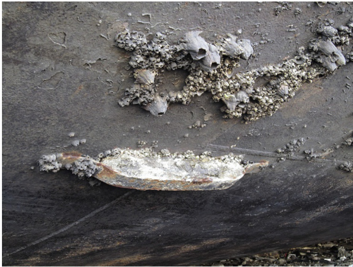
FIGURE 28.2 Magnesium sacrificial anode attached to the steel hull below the waterline.
