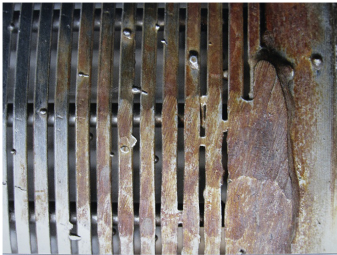
FIGURE 28.8 The stainless steel has rusted where it has been ground and machined.
