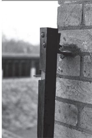
The crack path in a failed end post
