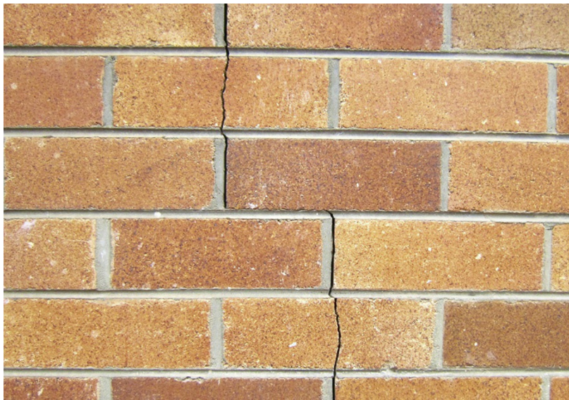
FIGURE 15.4 Brittle cracking of cement and bricks.
