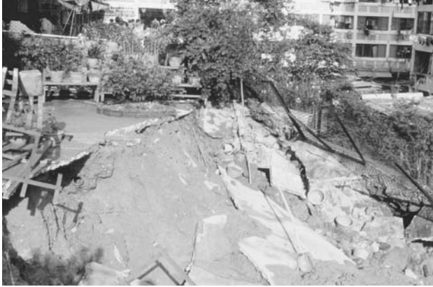
Figure 5.1. Small slope failure triggered by a burst water main – no injuries (Tsz Wan Shan, Hong Kong).
