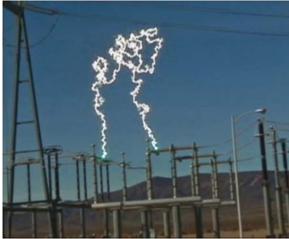
Figure 2.19 Arcing in a high-voltage switchyard (Source: http://www.lifeaftercoffee.com/2006/05/23/worlds-biggest-jacobs-ladder )
