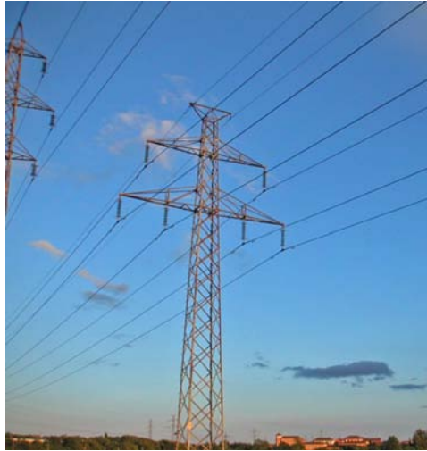
Figure 2.17 Typical high-voltage transmission lines (Source: http://commons.wikimedia.org/wiki/File:Electric_transmission_lines.jpg )
