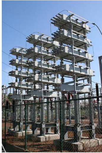
Figure 2.10 High-voltage capacitor banks (Source: http://en.wikipedia.org/wiki/File:Condensor_bank_150kV_-_75MVAR.jpg )
