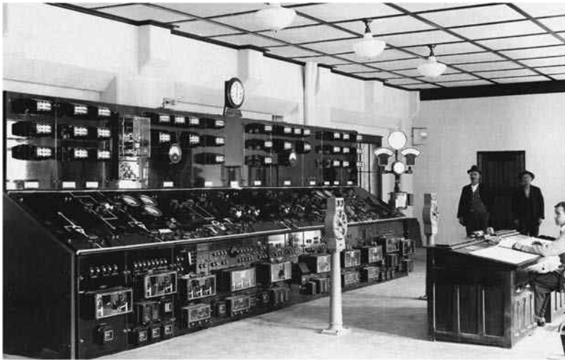
Control room of the Waikaremoana hydro station, New Zealand, 1928 (Source: Neil Rennie)
