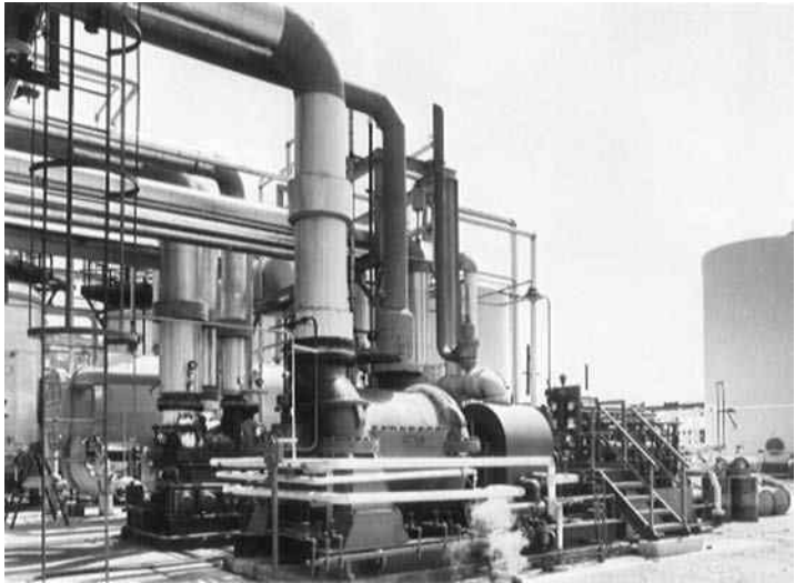
FIGURE 23.2 Multistage centrifugal compressor in a petrochemical plant. (Source: Elliott Company, Jeannette, Pa.)
