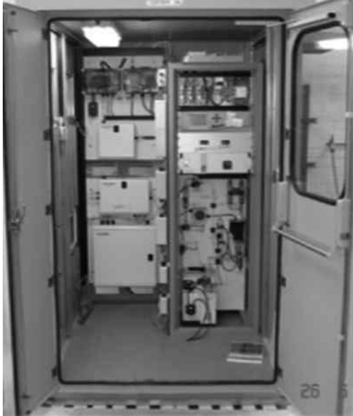
Figure 5.46 Typical extractive CEM. © Servomex, reproduced with permission
