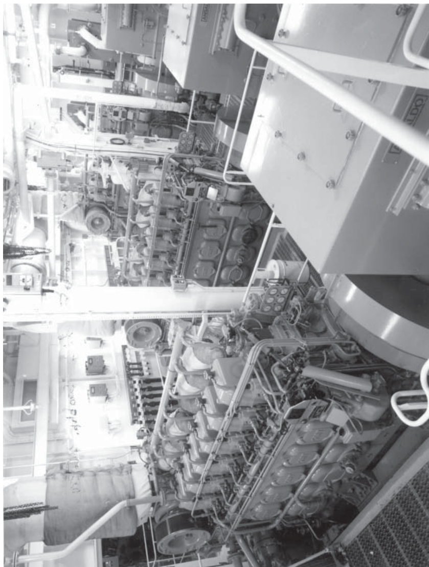
Figure 30.7 GMT BL230 engines in a genset installation
