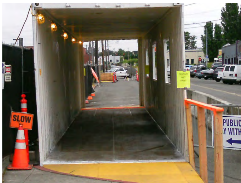
Figure 10-6: Example of Pedestrian pathway around construction sites (Picture Courtesy of Korsmo Construction)
