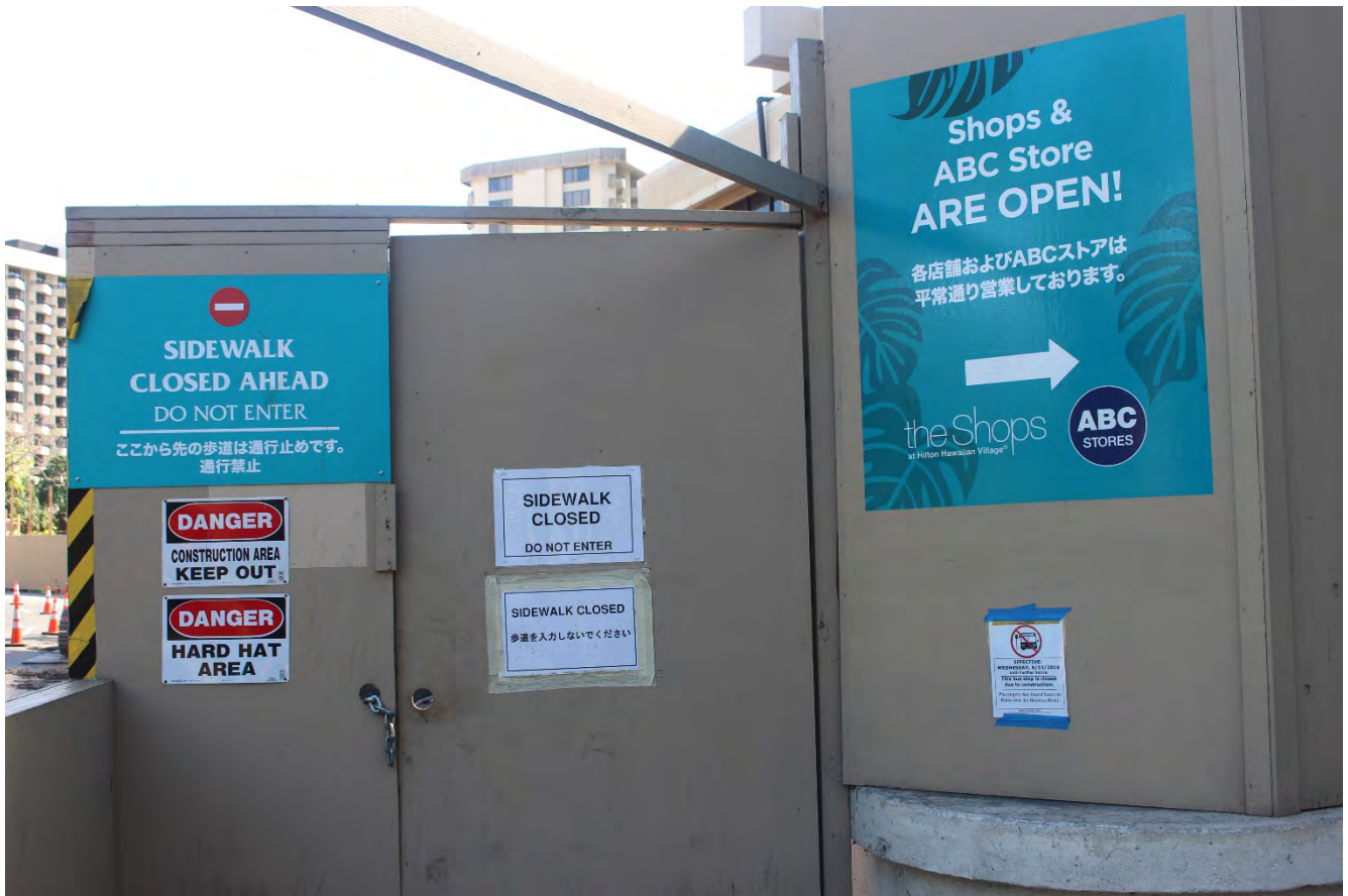
Figure 10-7: Example of Sidewalk Closed Signage and Barricade (Picture Courtesy of Hensel Phelps Construction)
