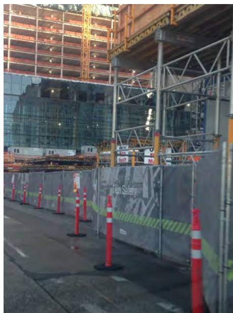
Figure 10-1: Example of Properly Installed Construction Site Security Fence (Picture Courtesy of Sellen Construction)
