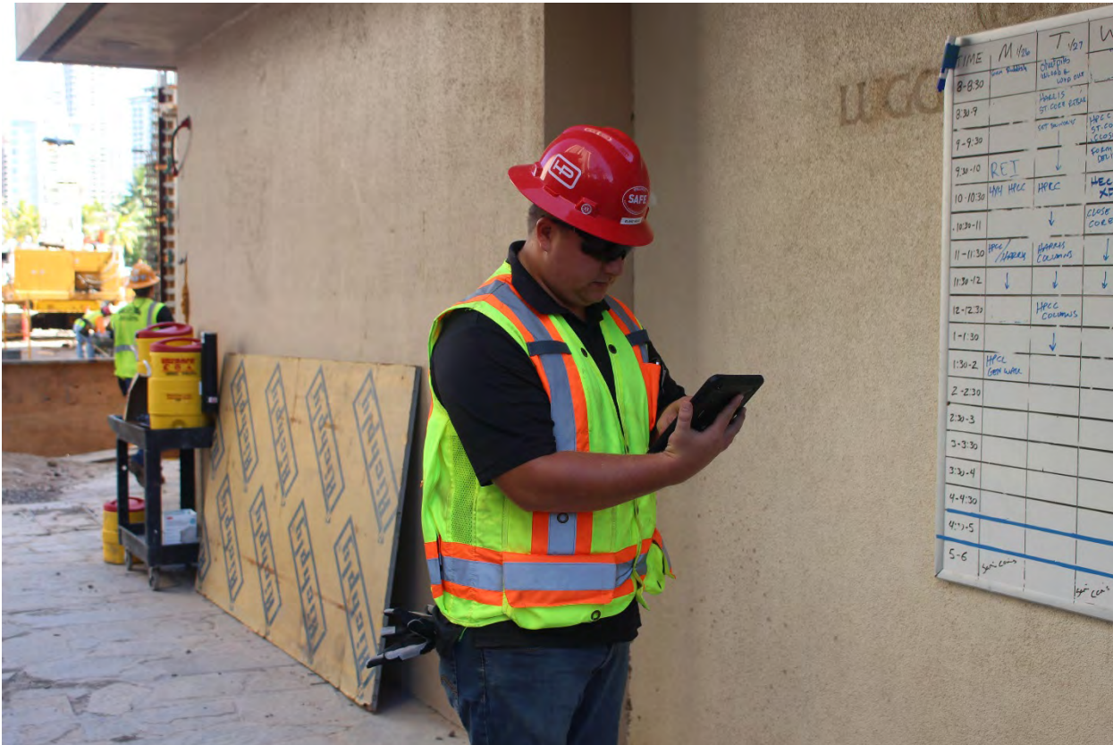
Figure 8-4: Safety Audit Using Smartphone Apps on an iPad (Photo courtesy of Hensel Phelps Construction)
