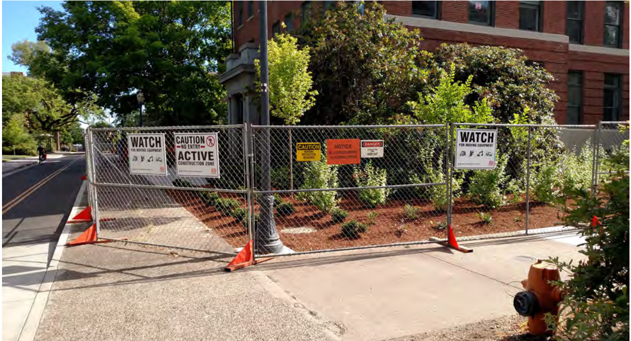
Figure 10-2: Example of Properly Installed Site Fence with Appropriate Warning Signage (Picture Courtesy of Hoffman Construction Company of Oregon).
