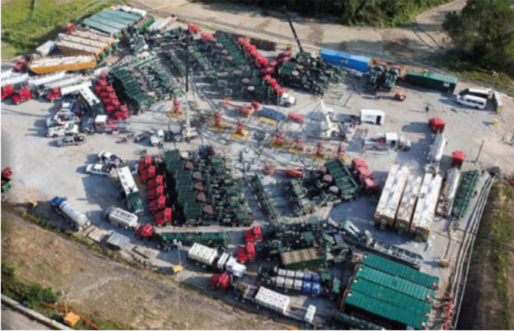
Figure 17.13 Photograph of hydraulic fracturing site with two wellheads. Source: NETL (2011).
