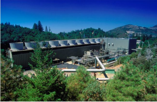
Figure 13.17 One of the Geysers hydrothermal power plants (NREL 17270). Source: http://images.nrel.gov/viewphoto.php?imageld=6318101 .
