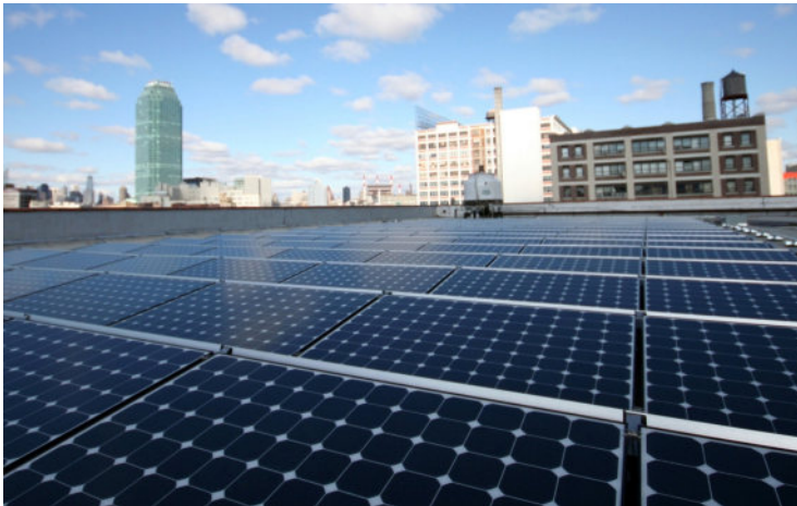
Figure 9.16 A 49 kW photovoltaic array. Source: http://images.nrel.gov/viewphoto.php?imageId=6322492 .
