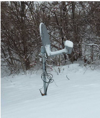
Figure 4.6: A snow covered dish antenna.
