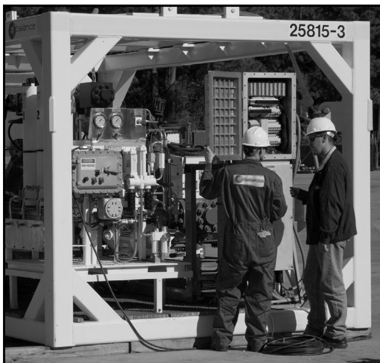
Figure 3.11 An open PLC on the DAPC choke manifold. The PLC contains the safety-critical control technology that manages the manifold's operation.
