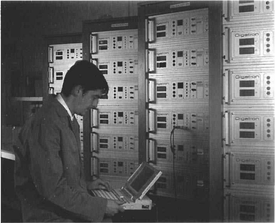
Fig. 12.27 Computer monitoring of cell voltages (courtesy of Invensys)
