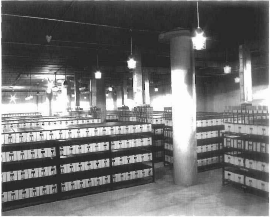
Fig. 12.29 Typical battery installation (courtesy of Invensys)
